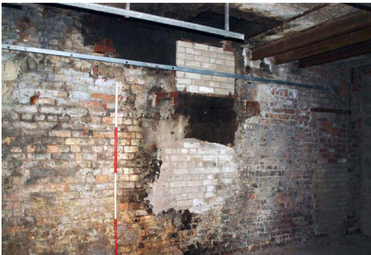
Plate 33. 'B' Mill, basement, on opposite side of wall from Plate 32, showing cast-iron wallbox with damaged bracket; above this is a cast-iron trap built into ceiling. Viewed from south-west (by S. Price).
