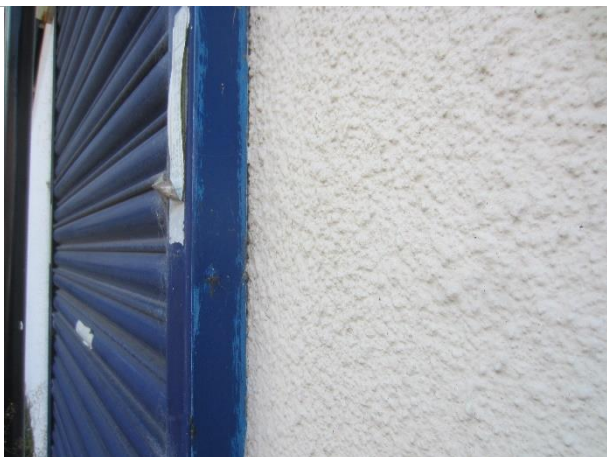
Photo 7: Sealed door and window apertures
