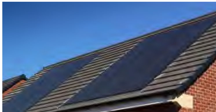
Inline photovoltaic panels (solar panels)
