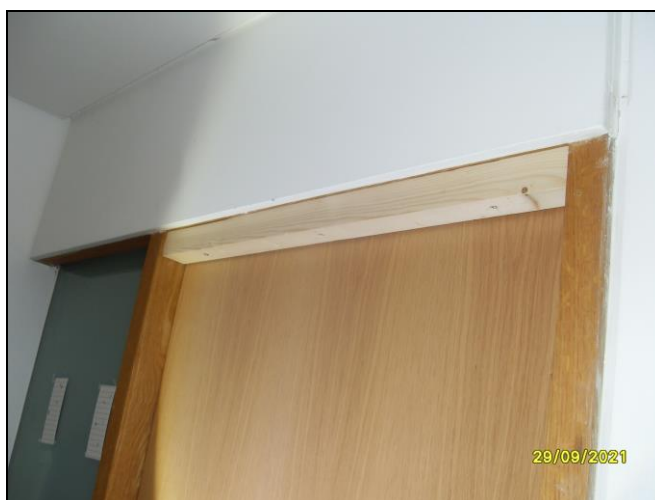
Insufficient fire-stopping to fire door
