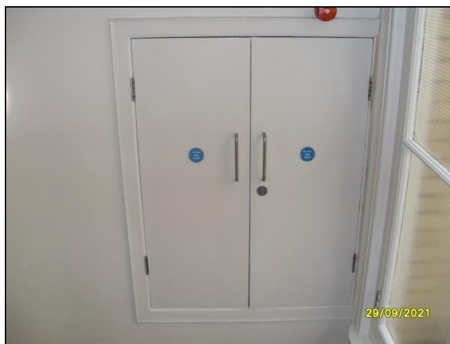
Riser doors scheduled for replacement
