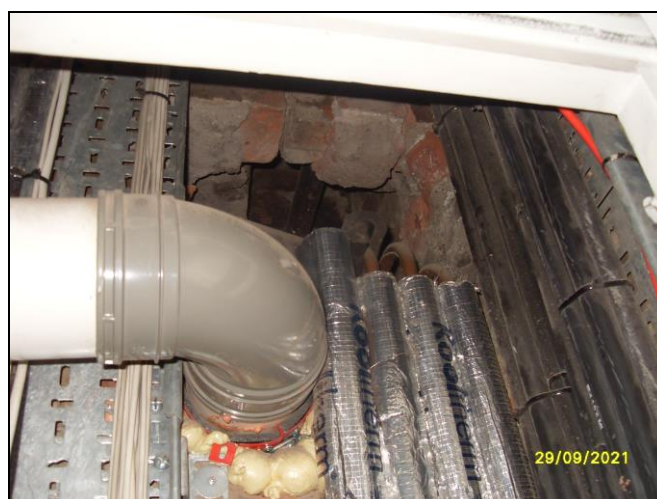
Poorly fire-stopped service penetration
