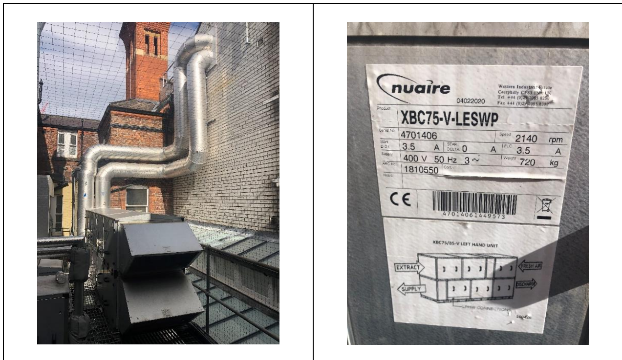
Existing AHU serving the Council Chamber
