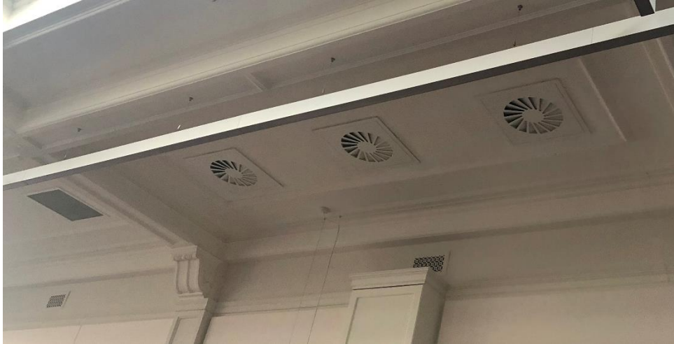
Existing supply and extract diffusers in Council Chamber ceiling
