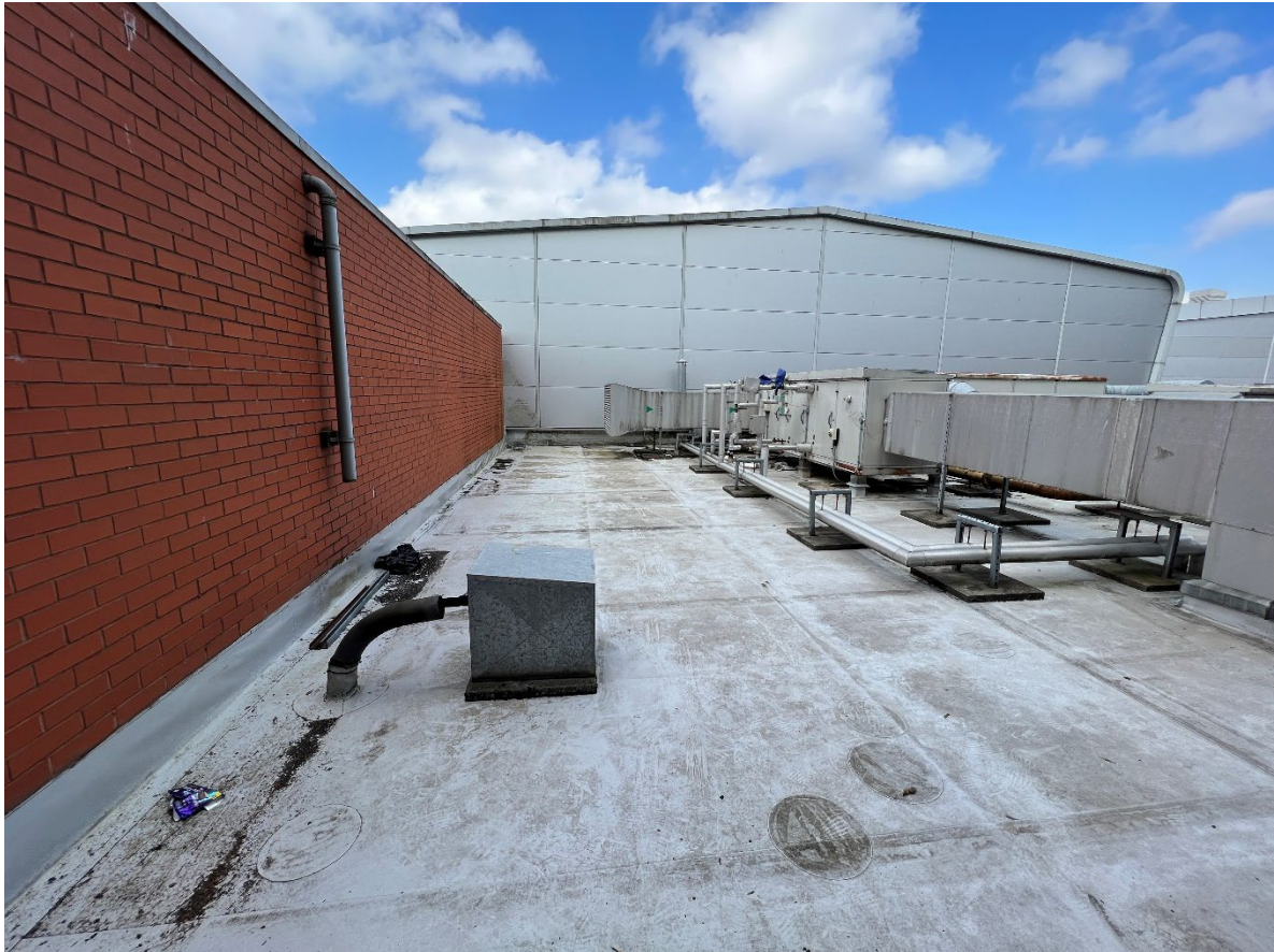
Photograph 5: The DHW ASHP to be located on the roof, this will not be visible at ground level.
