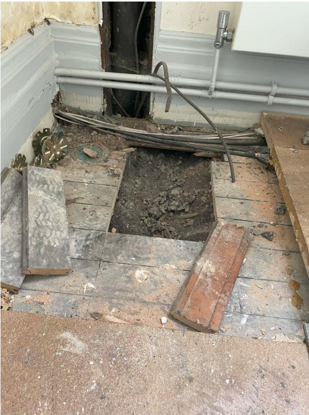
Shallow plywood raised access floor and damage to timber floor
