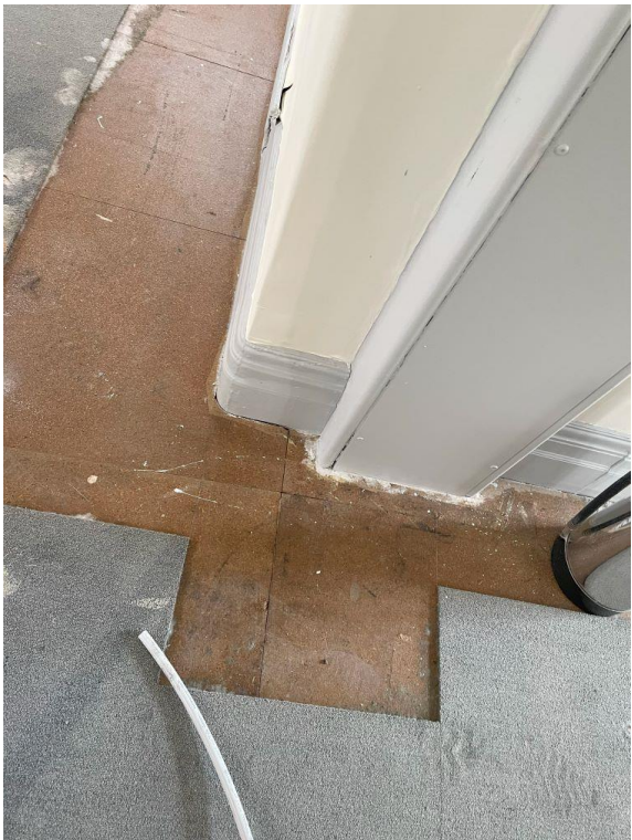
Raised access floor
