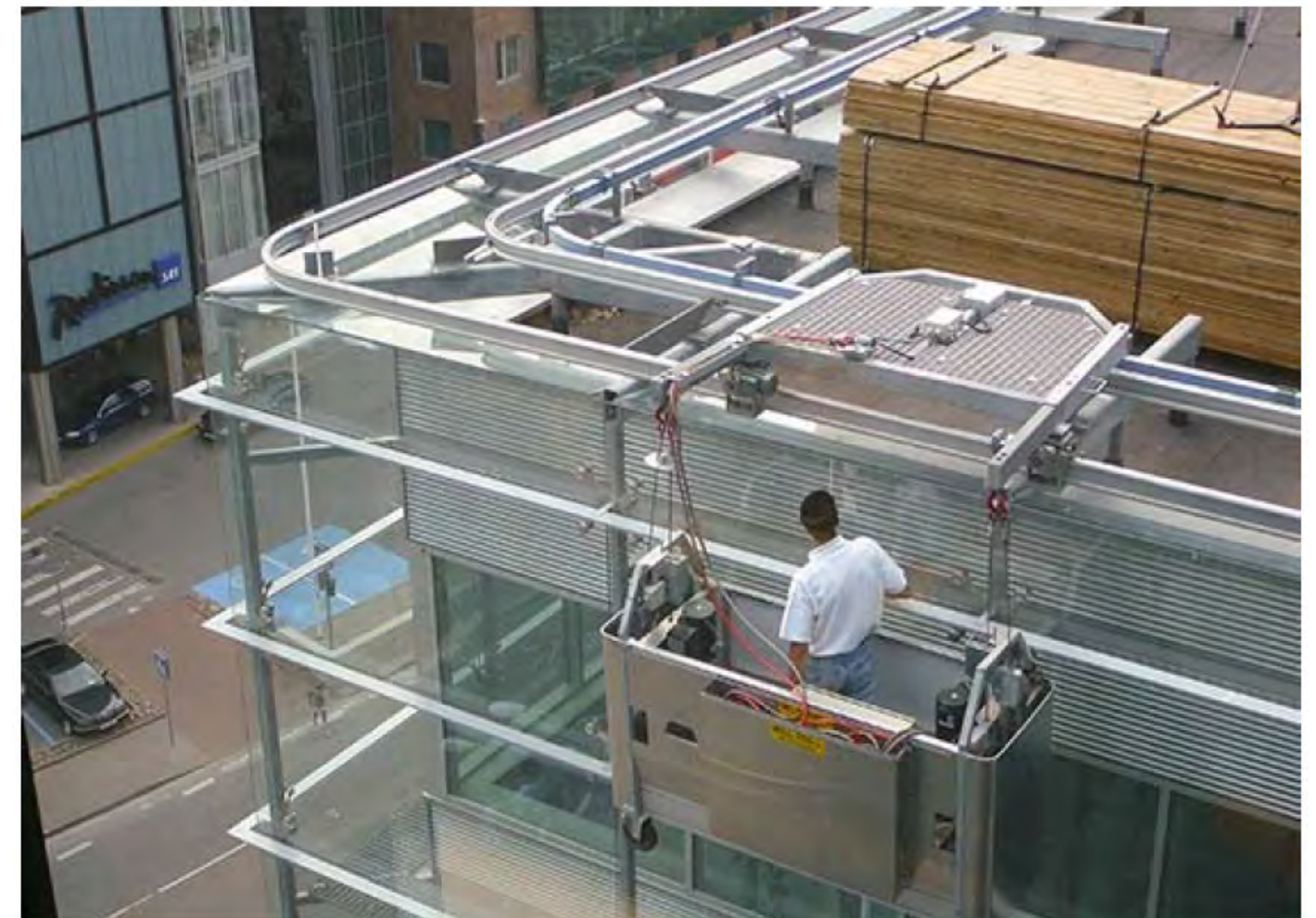
Example of roof trolley and cradle system
