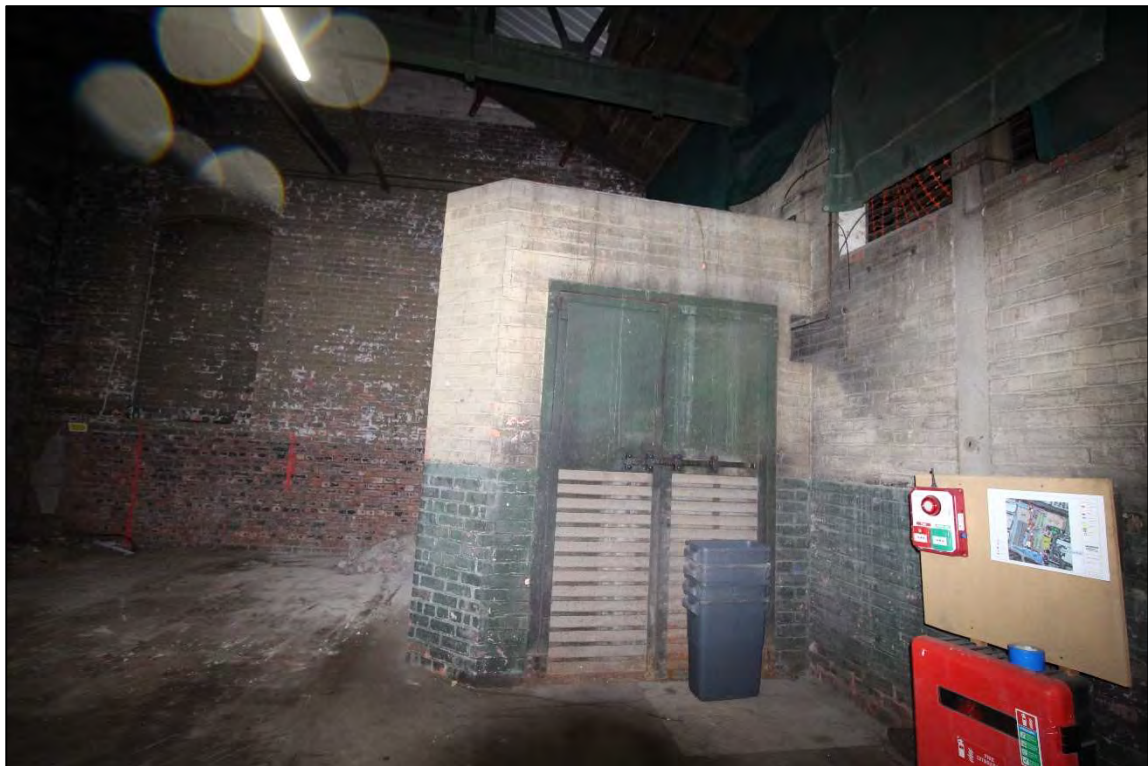
Plate 33: General view of the live electrical area, Room 2
