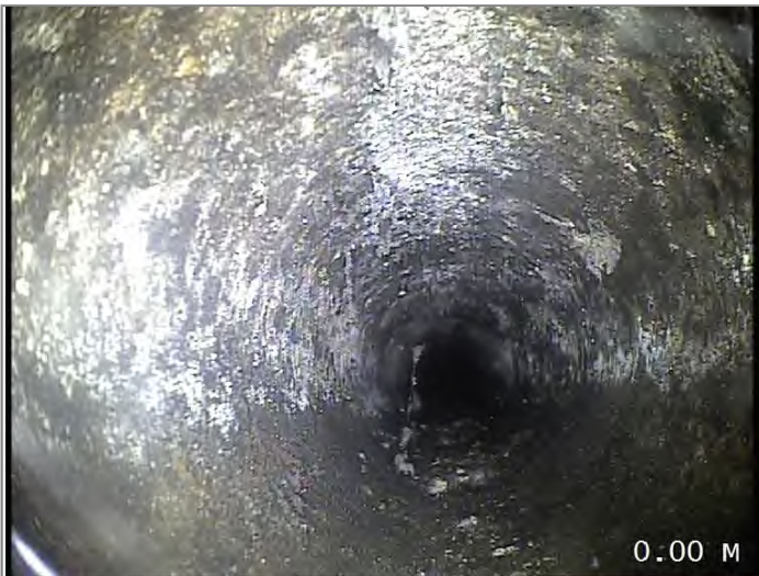
Start node type, manhole, reference MH9
