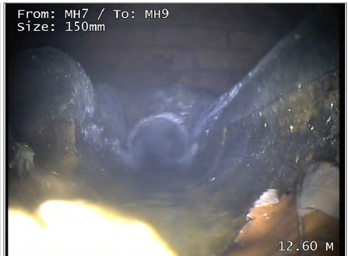
Finish node type, manhole, reference MH9
