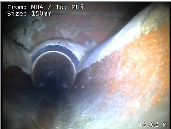
Finish node type, manhole, reference MH5
