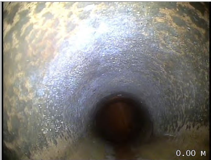
Start node type, manhole, reference MH3
