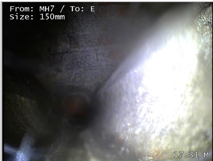
Finish node type, manhole, reference MH10
