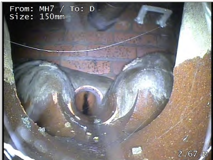
Finish node type, manhole, reference MH8
