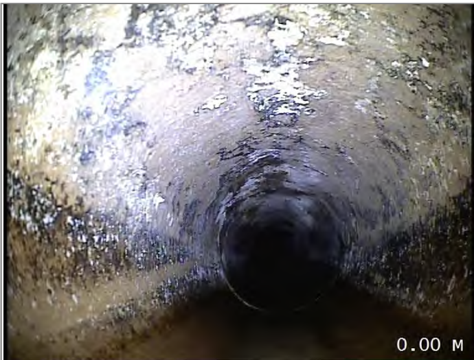
Start node type, manhole, reference MH1
