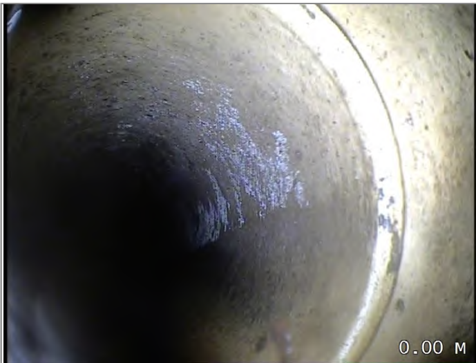
Start node type, manhole, reference MH22
