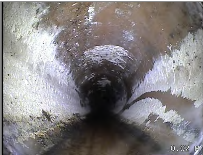
Start node type, manhole, reference MH13
