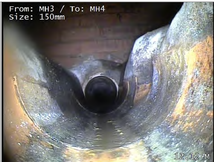
Finish node type, manhole, reference MH4
