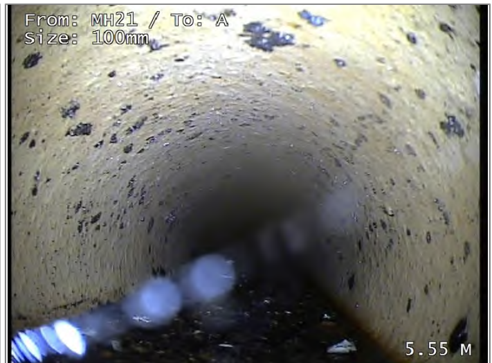
Survey abandoned - Remark: DUE TO SILT IN LINE
