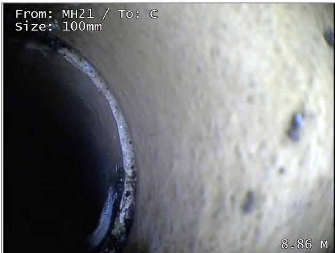
Line of drain/sewer deviates left
