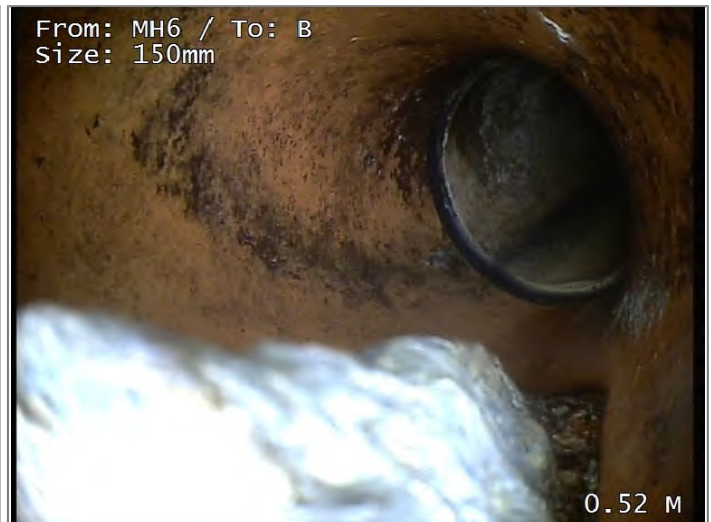
Survey abandoned - Remark: CONCRETE IN LINE
