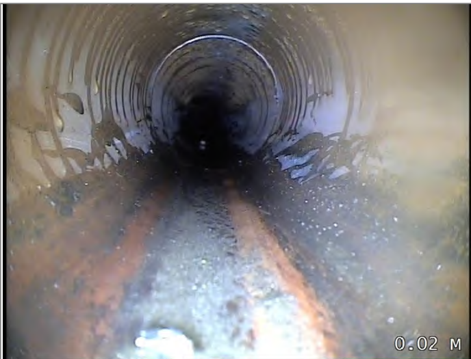
Start node type, manhole, reference MH29
