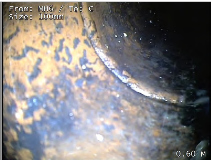
Line of drain/sewer deviates right
