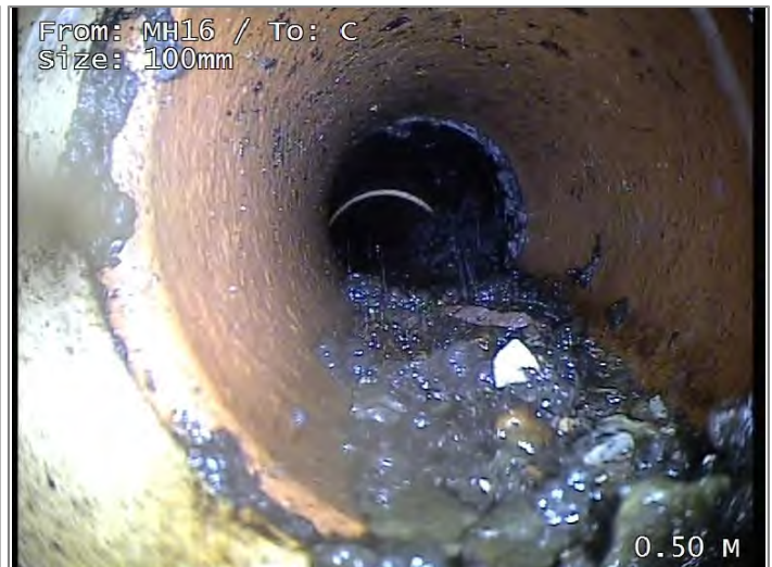
Survey abandoned - Remark: DUE TO DER
