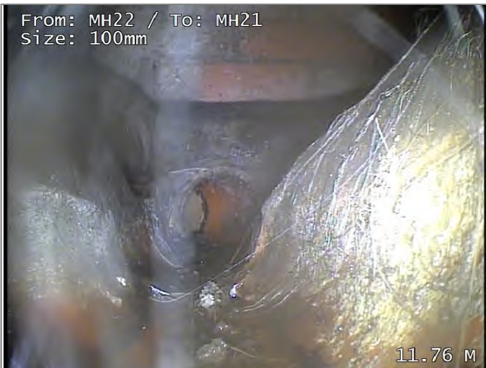
Finish node type, manhole, reference MH21
