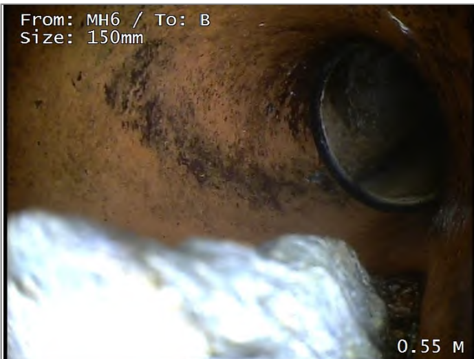
Settled deposits hard or compacted 20% cross-sectional area loss
