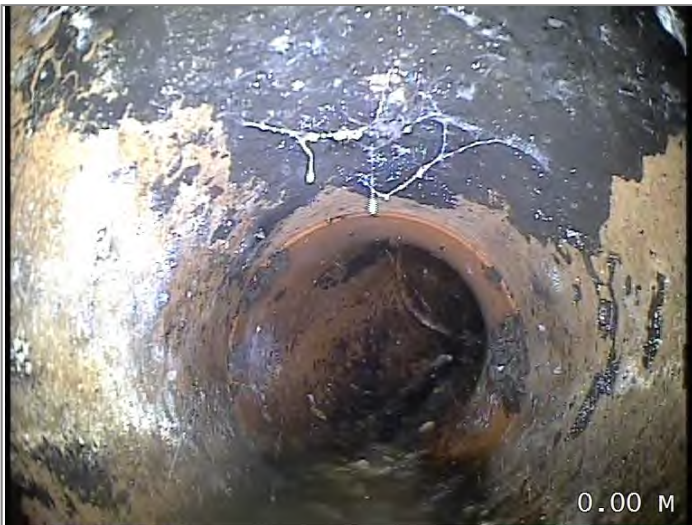
Start node type, manhole, reference MH6
