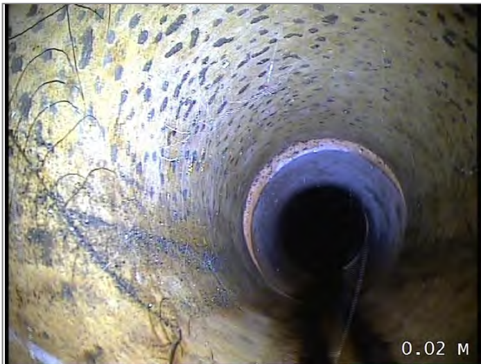
Start node type, manhole, reference MH7
