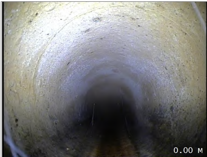
Start node type, manhole, reference MH21
