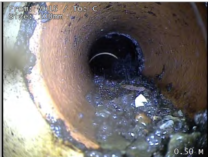
Settled deposits coarse 15% cross-sectional area loss
