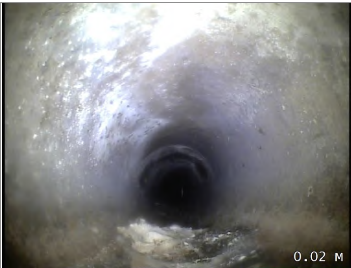
Start node type, manhole, reference MH4
