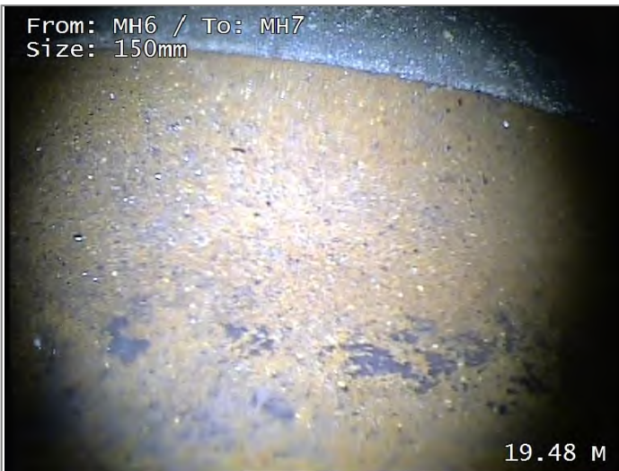
Finish node type, manhole, reference MH7
