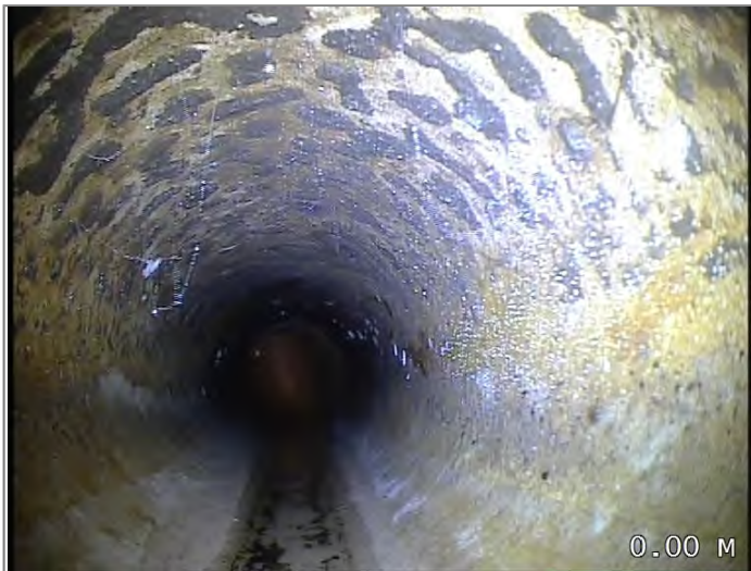
Start node type, manhole, reference MH7
