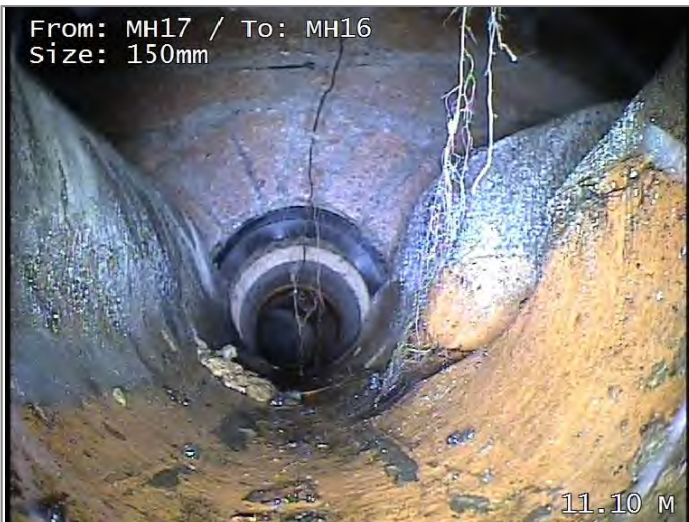
Finish node type, manhole, reference MH16
