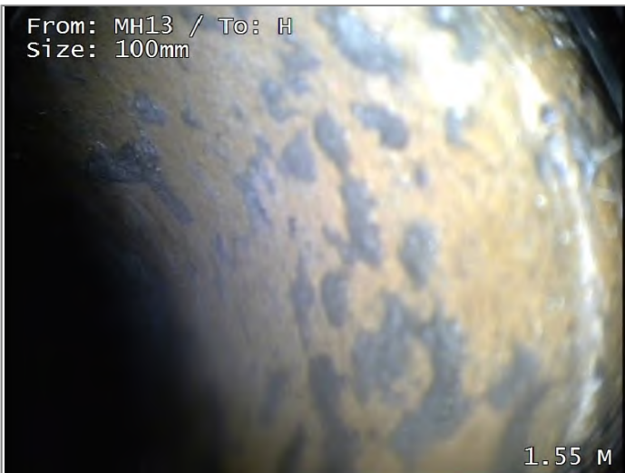
Line of drain/sewer deviates left
