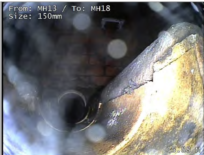
Finish node type, manhole, reference MH18
