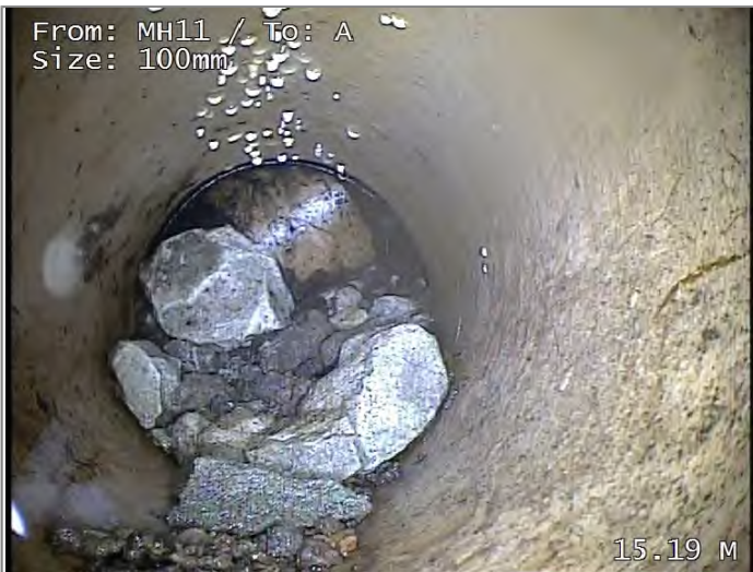
Settled deposits coarse 25% cross-sectional area loss
