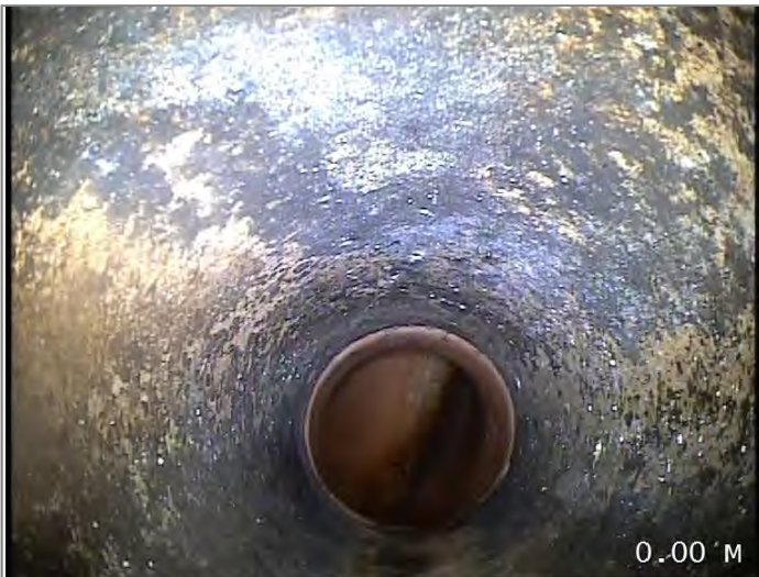
Start node type, manhole, reference MH3
