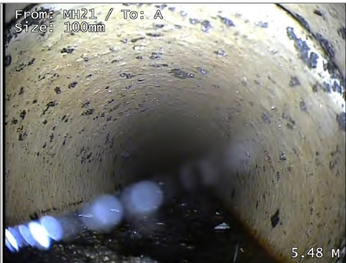
Settled deposits fine 15% cross-sectional area loss
