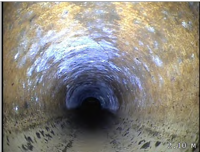
Start node type, manhole, reference MH20
