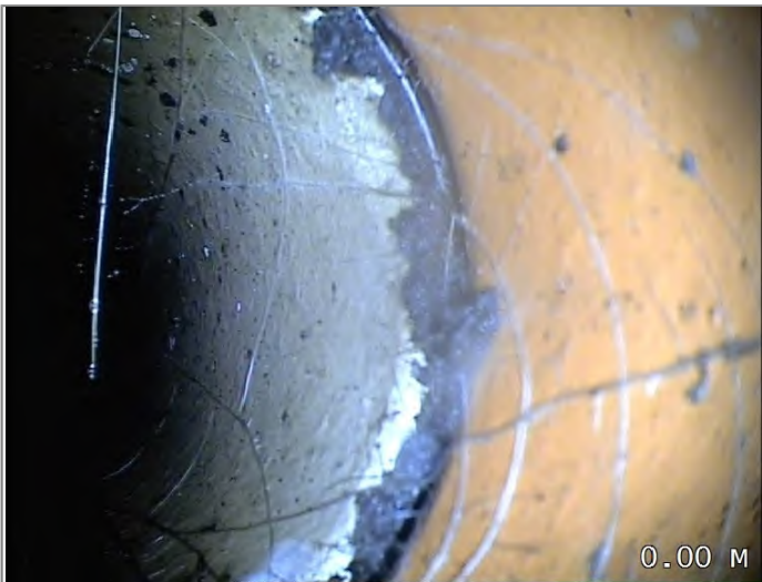
Start node type, manhole, reference MH21
