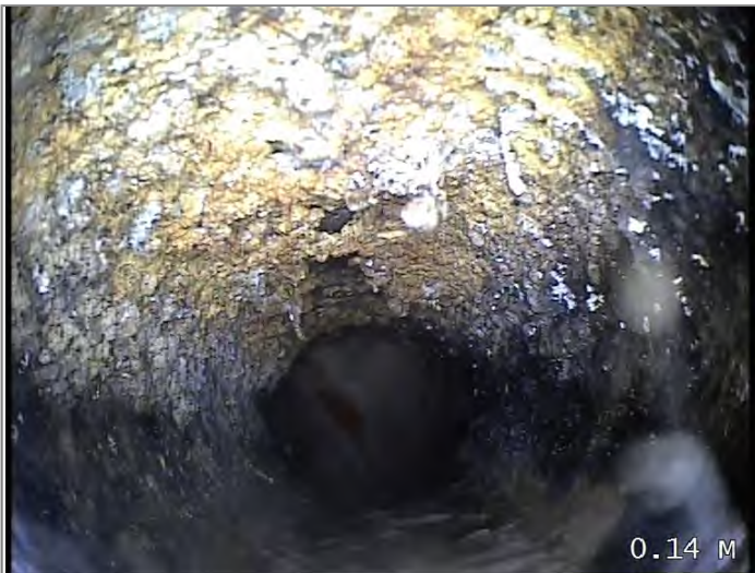
Start node type, manhole, reference MH13
