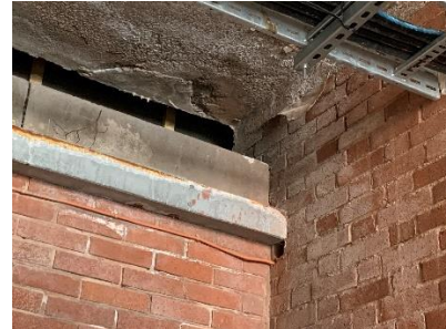
Photograph 3 – A small void found down the exterior service ramp
