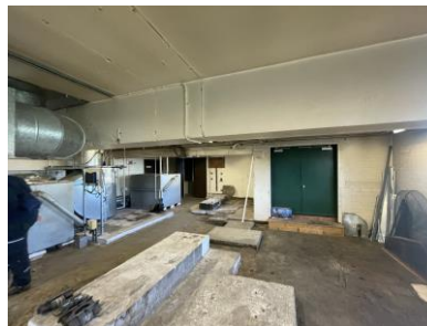
Photograph 7 – Central plant store room
