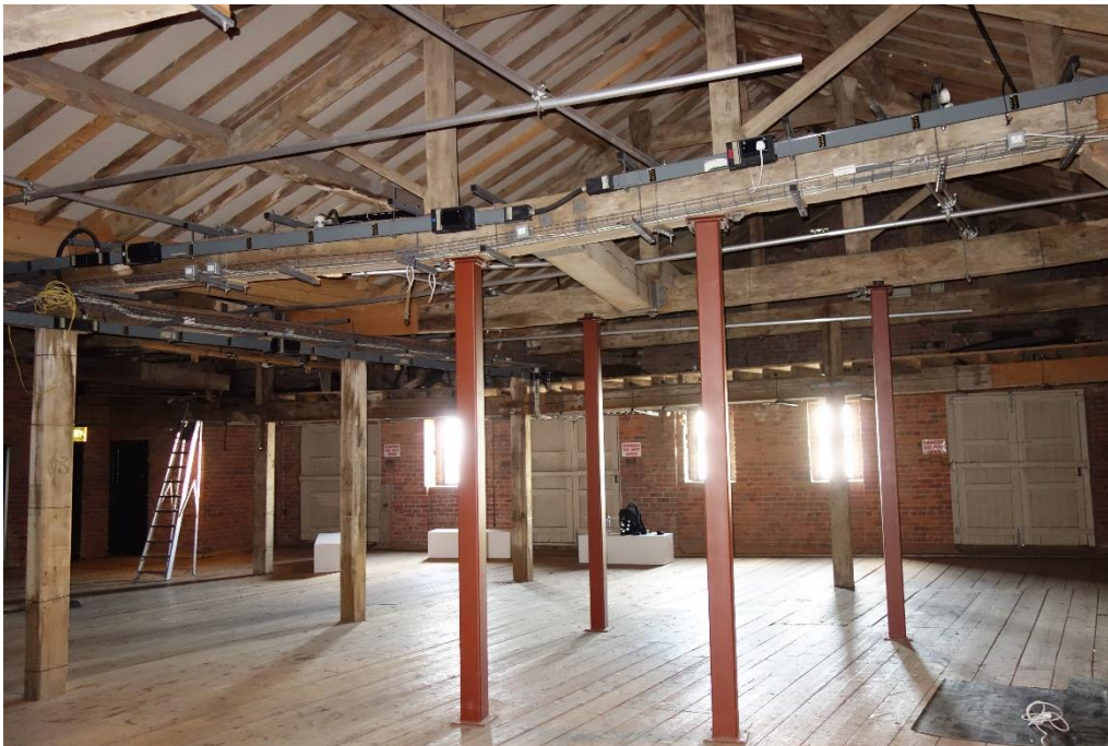
Photograph 1: General view of propped failed trusses in Bay 2.
