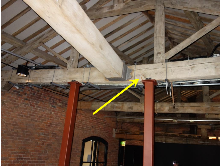
Photograph 2: Detail view of damaged truss chord. The crack location is arrowed.
