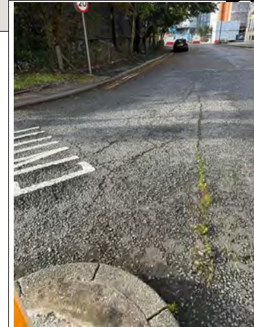
Additional photo taken 13/10/2023 indicating clearer evidence of longitudinal and transverse cracking in this location in dry conditions.
