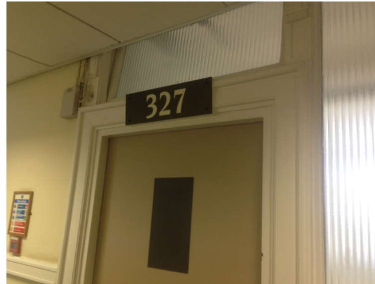
uncomfortable junctions between joinery, reeded glass and ceiling
