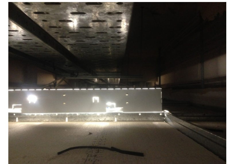
cable trays and recessed lighting
