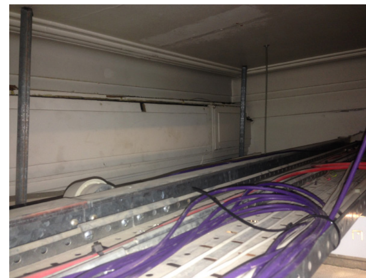
large ceiling voids, compromising height of offices and concealing extensive cabling within ceiling void
