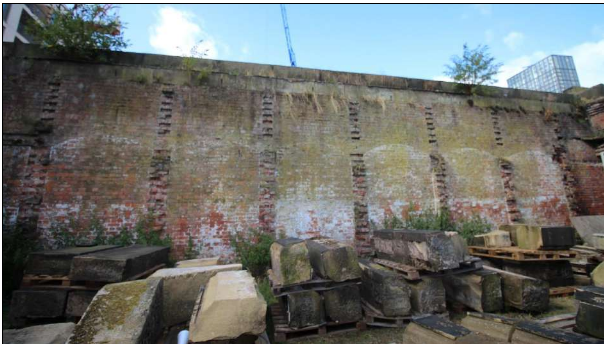
Plate 36: Detail of the wall scars at the south-eastern end of the south-west wall
