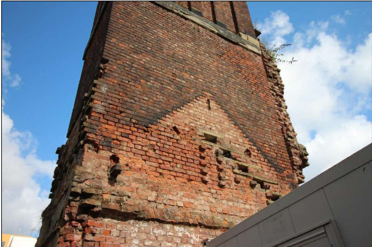
Plate 33: Detail of the scarring to the south-east elevation of the chimney
