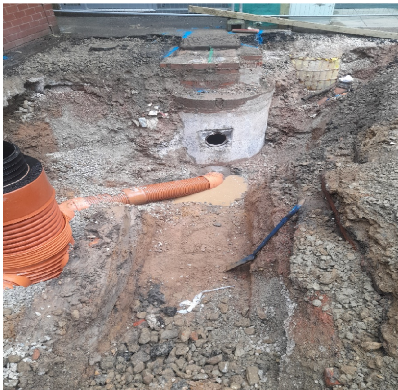
Photograph J (taken via Dave Shacklady J Greenwood (Builders) Limited) – Image taken west of site facing north. Image showing the natural ground and drainage in the location of WS1 following the clients removal of soils in the area.
