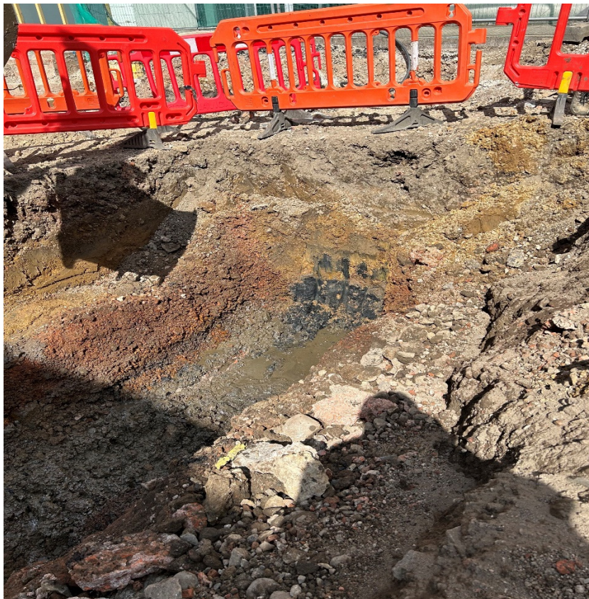
Photograph F – Image taken south of site facing north west. Image showing the resulting hydrocarbon impacted soils after the removal of the tank.
