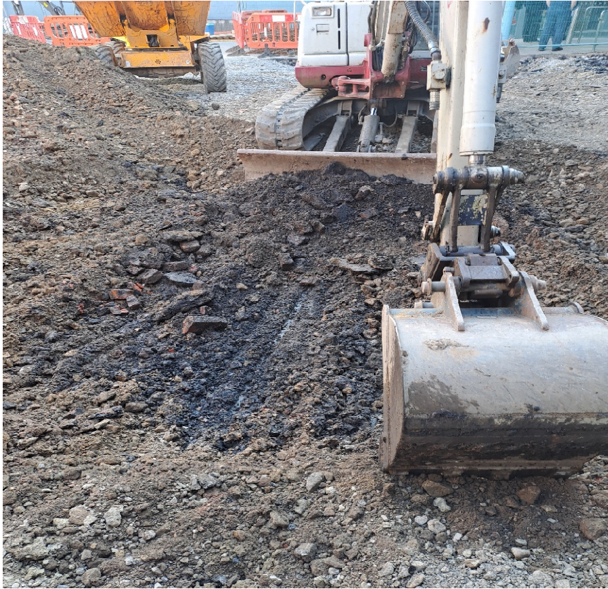
Photograph A – Image taken in the south western corner of the site facing east. Image showing black hydrocarbon staining within the Made Ground soils on site, subject to excavation.
