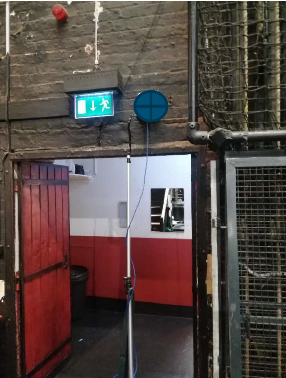
Location AP 6 - Stage right wings - Unit installed on the stage to provide full coverage. This unit would be clustered with other wall mounted technical equipment and painted black. Any fixings back to the original brick would minimize damage and allow for easy replacement in the future.
