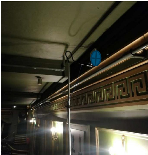
Location AP A15 - Stalls level - unit installed discreetly above cornice line. Conduit obscured.
