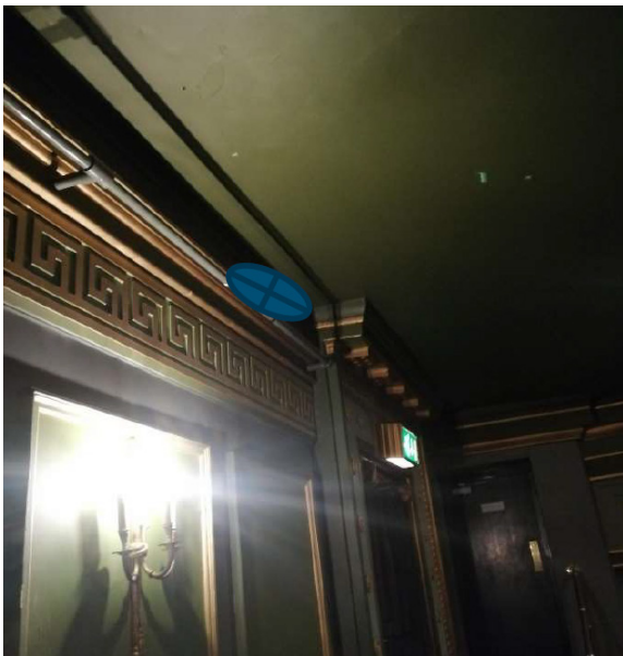
Location AP A6 - Stalls level - unit installed discreetly above cornice line. Conduit obscured.
