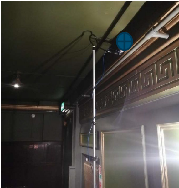
Location AP A12 - Stalls level - unit installed discreetly above cornice line. Conduit obscured.
