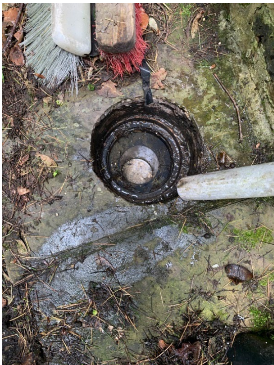
Photo 1 (Unable to remove FWG1 trap without breaking it to survey)
