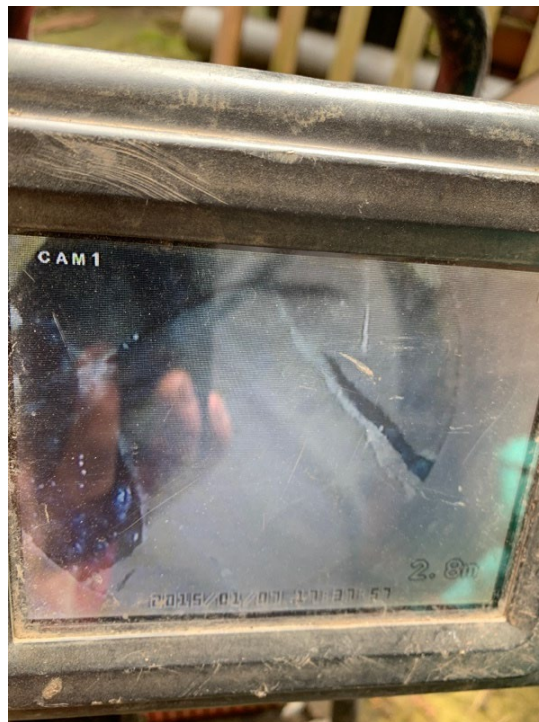
Photo 2 (SVP downstream large break in pipe at 2.90m)
