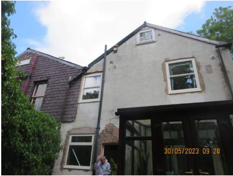
Rear elevation, showing render deterioration
