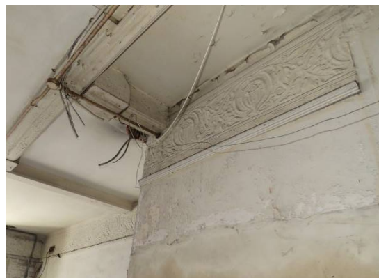
Figure 9: An area of Victorian embossed paper frieze, originally located in the ground floor level of The Site, and since removed.
