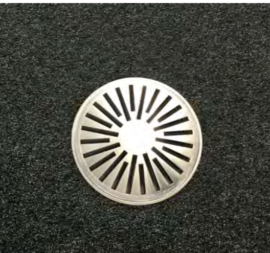
Q200 SUPPLY AIR DUCT RISES FROM BELOW TO SERVE SWIRL DIFFUSER.
