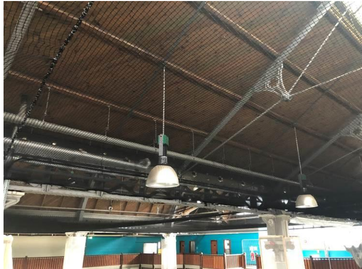
Figure 62: The south-east corner of the roof structure, showing the 1980s timber boarding replacements and modern lights.
