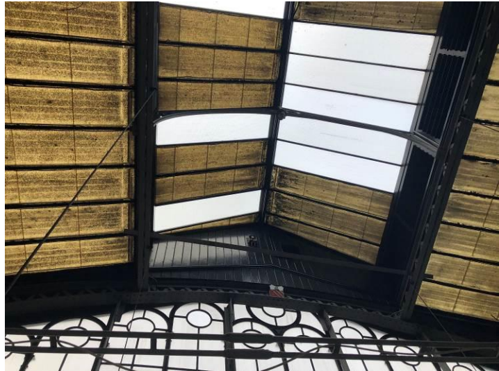
Figure 64: An example of the modern 1980s fibreglass panels (discoloured) and more recent clear coverings.
