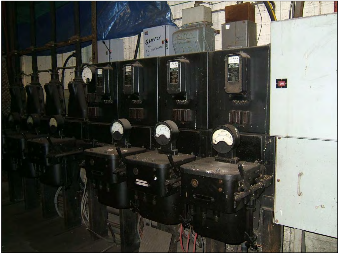
Plate 103: The original electrical equipment to the northern end of Room 3
