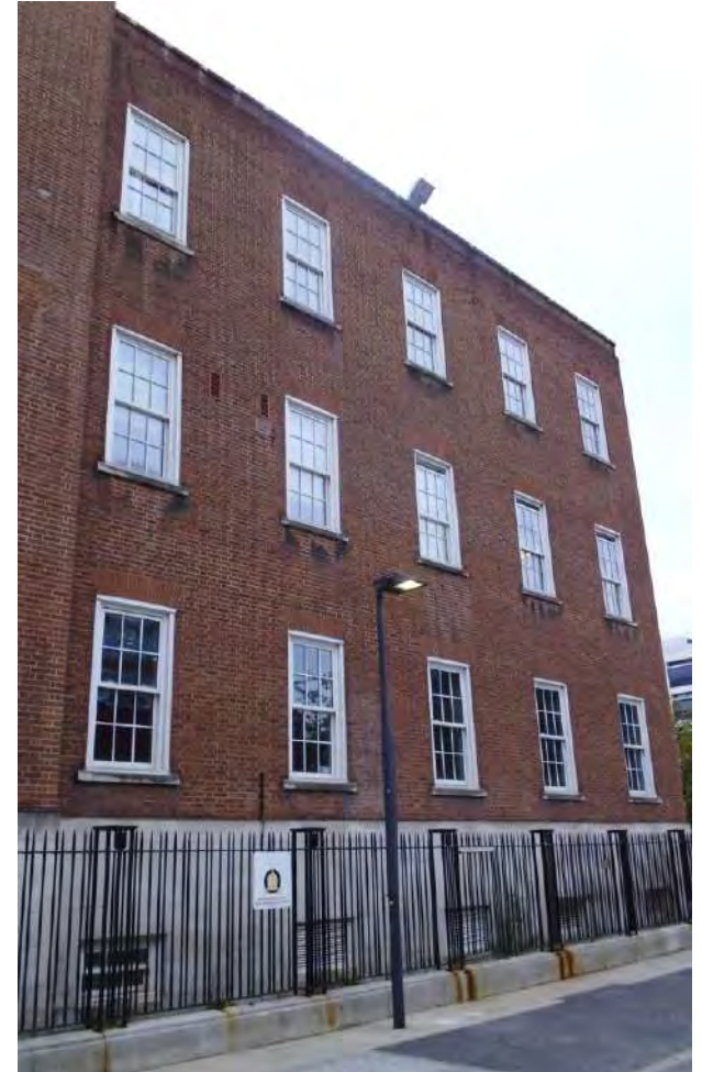
Example of staining to brick façade beneath cills
