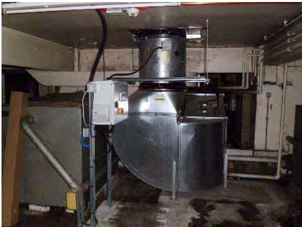
Live kit in Plant Room of Zochonis Building
