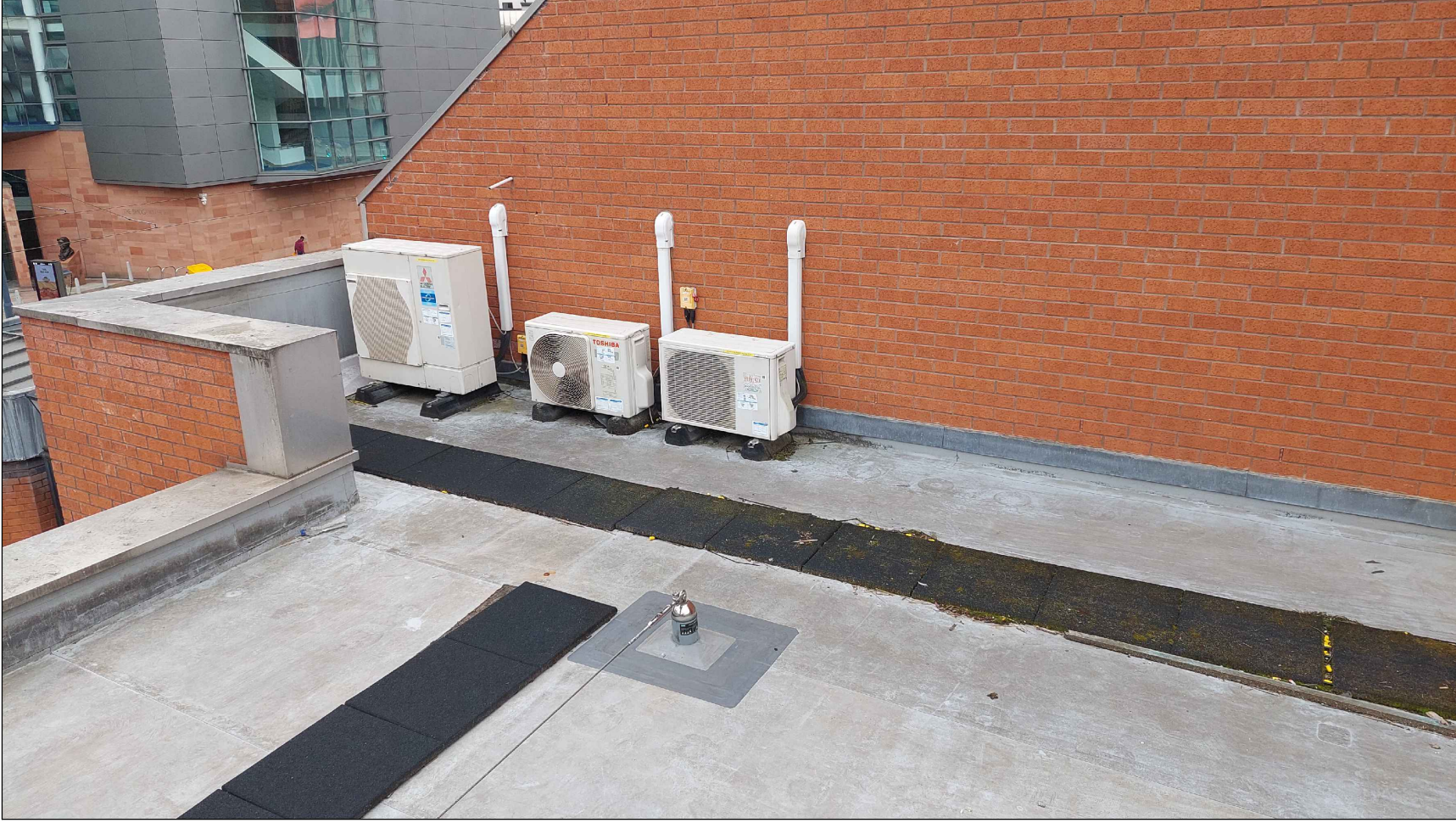
PHOTO 8 – EXISTING 3NO. CONDENSERS SERVING FIRST FLOOR OFFICES.
