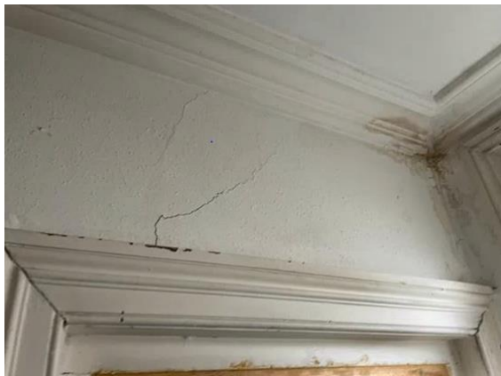
Crack in hallway
