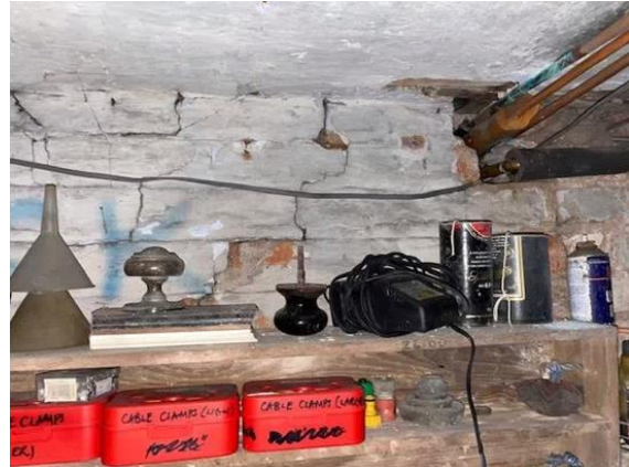
Crack in cellar wall.
