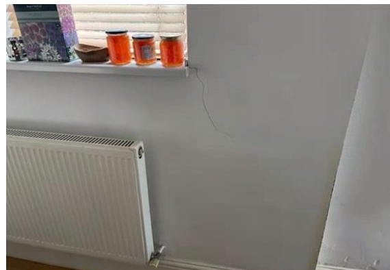
Crack in rear dining room
