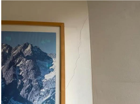
Crack in rear dining room
