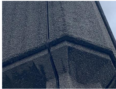
Photograph 2 – Close-up on the ridges between concrete
