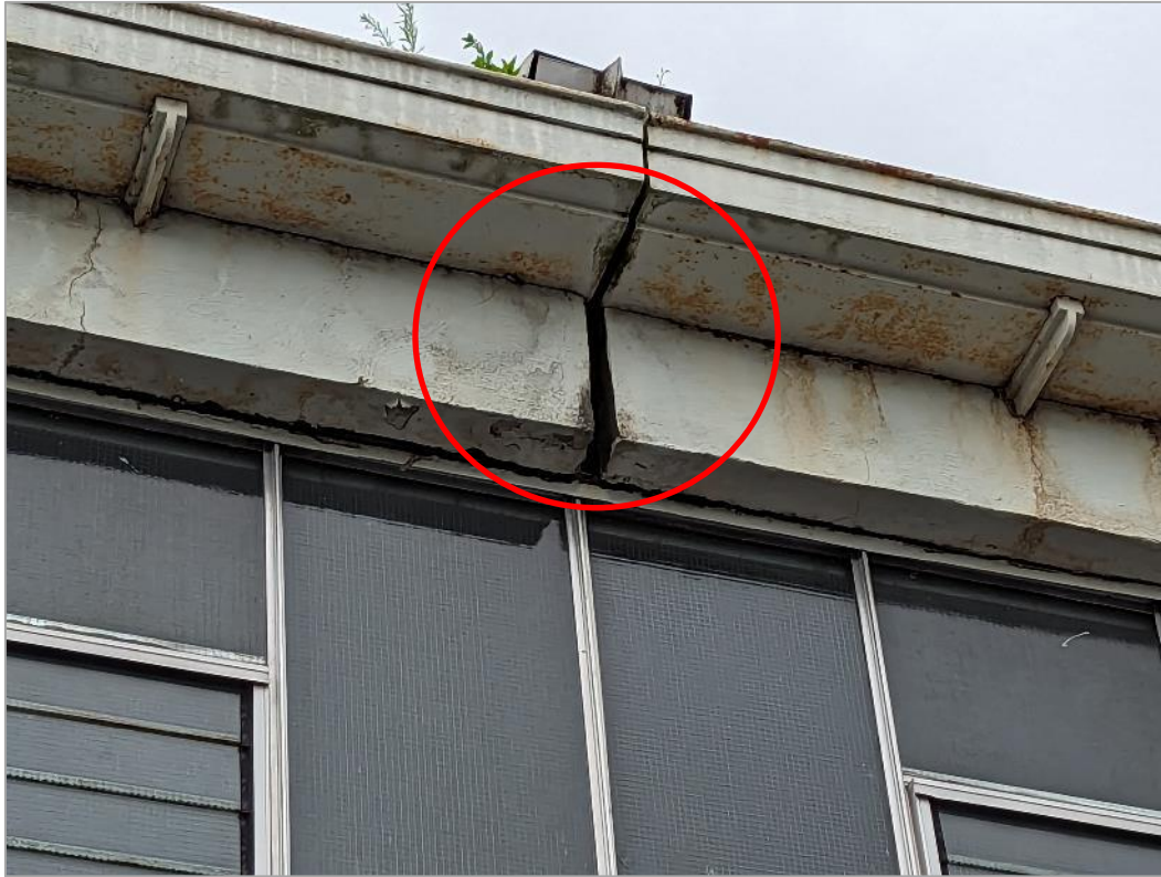
Plate 8 – Large crack in concrete slabs above window eastern aspect
