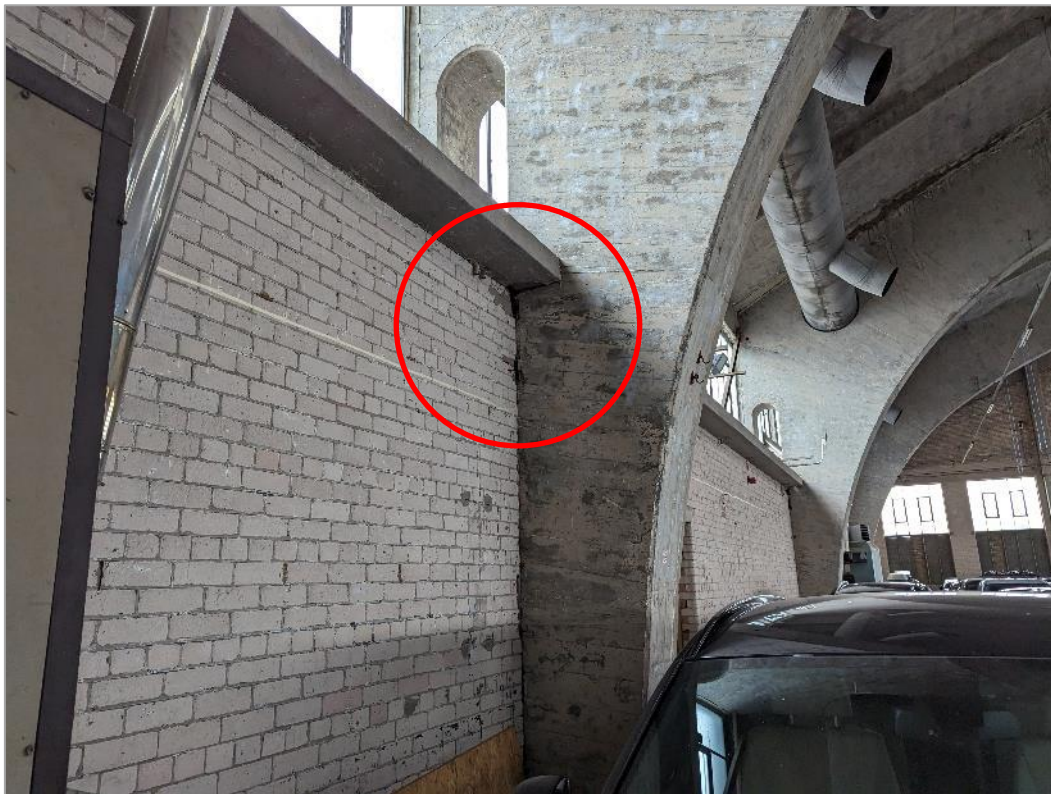
Plate 4 – Cavities / ingress opportunities in most areas of concrete arch / brick interface
