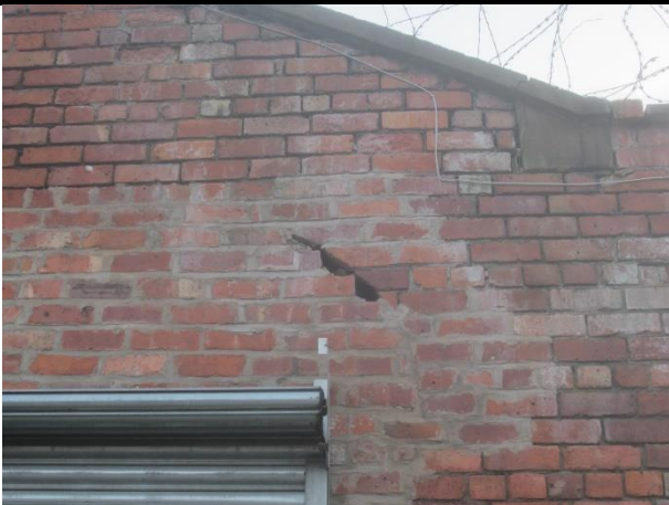
Photo 25: Holes in brickwork at eastern elevation of B4
