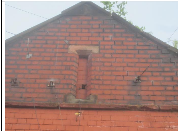
Photo 11: Gaps in the brickwork at the northern elevation of B2
