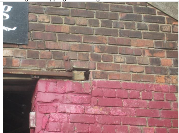
Photo 16: Holes in brickwork at B3 (western elevation)
