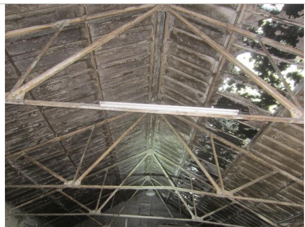
Photo 18: Interior of B3 showing uninsulated and unlined roof covering
