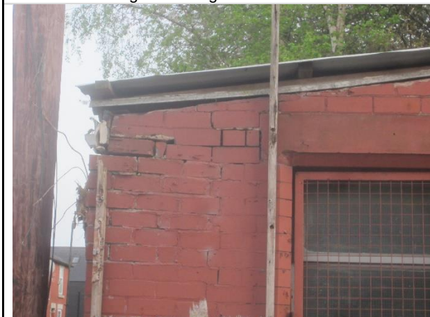
Photo 9: Gaps in brickwork and roof verge at northern elevation of B2
