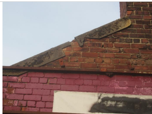
Photo 15: Gaps behind overlapping sheeting / fascia at western elevation of B3
