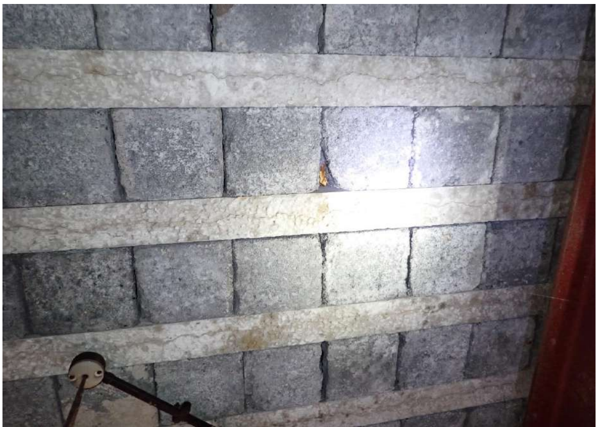
Photograph 12 – showing gaps between the blocks in roof access building.
