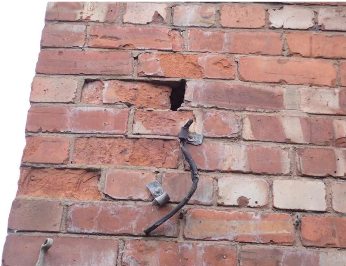
Photograph 8 – wall cavity PRF on north aspect.
