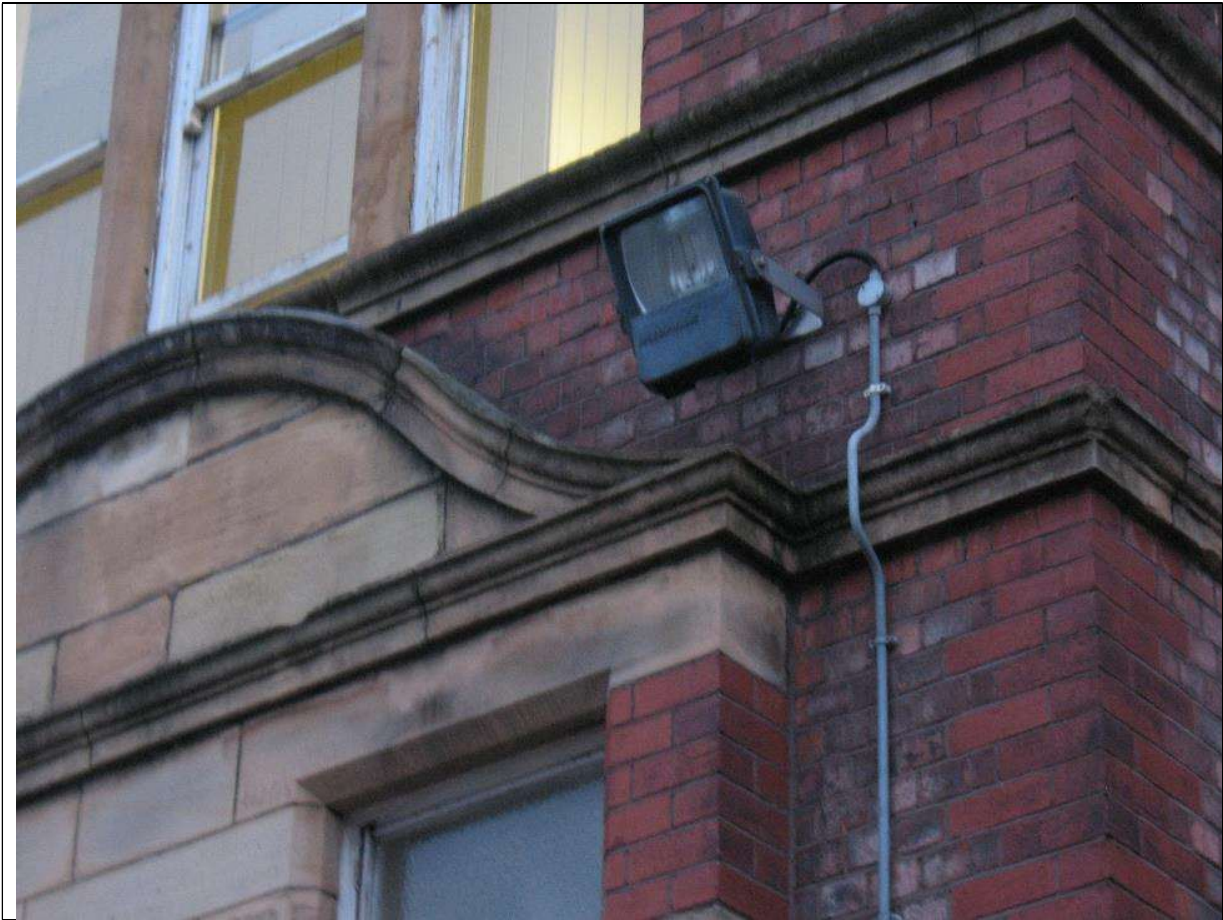
Photograph: 2 - Existing halogen floodlight installed on building exterior
