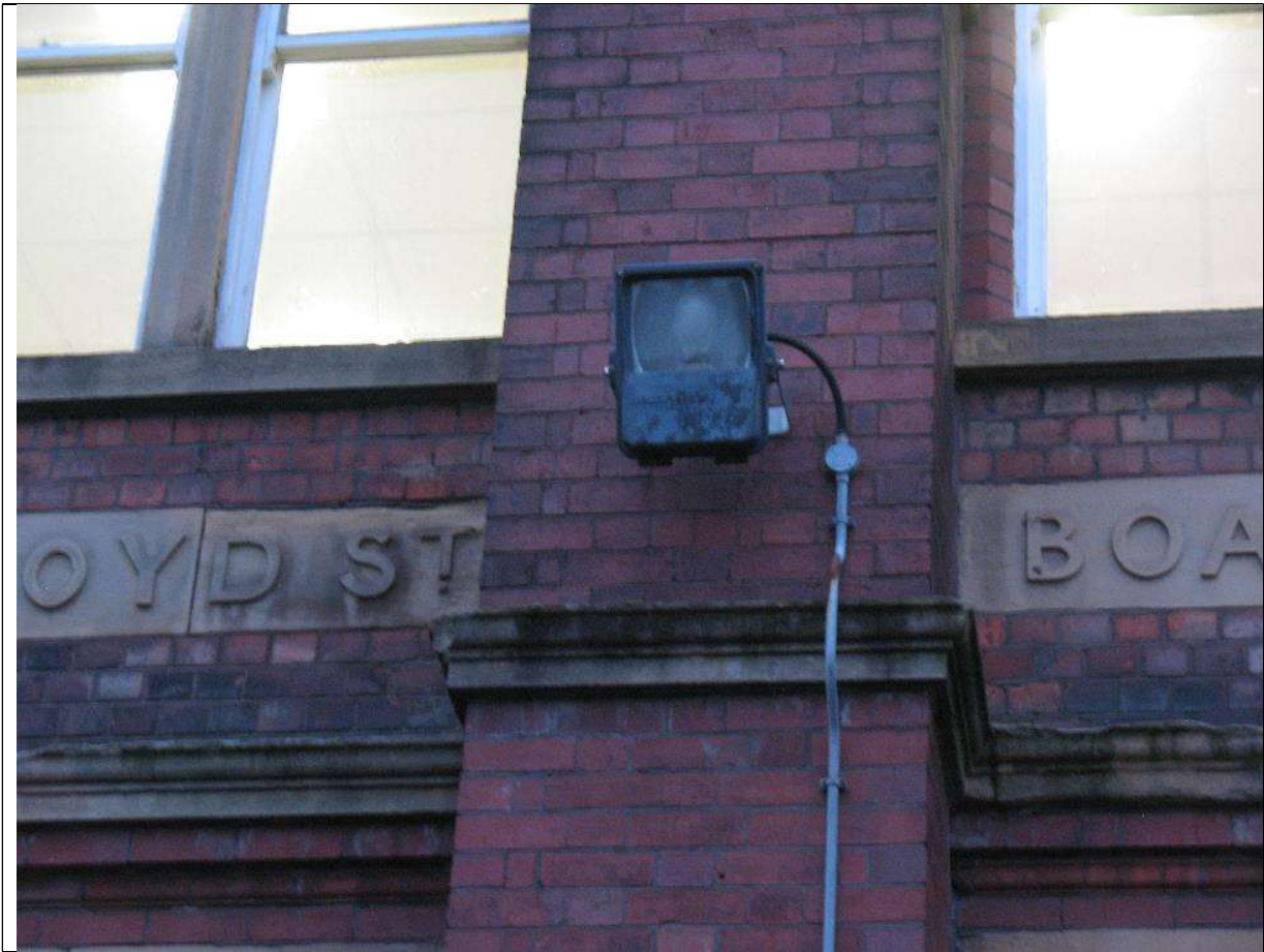
Photograph: 1 - Existing halogen floodlight installed on building exterior
