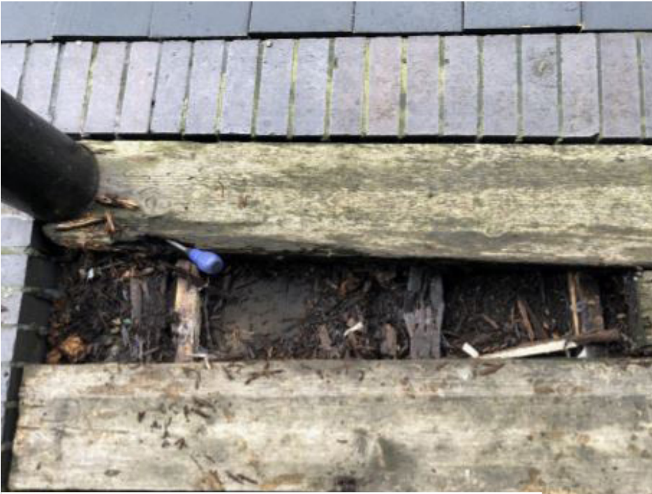
Wet rot decay to timber battens and boarding to platform boarding
