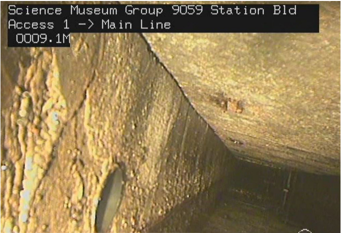
Typical outlet from Station Building
