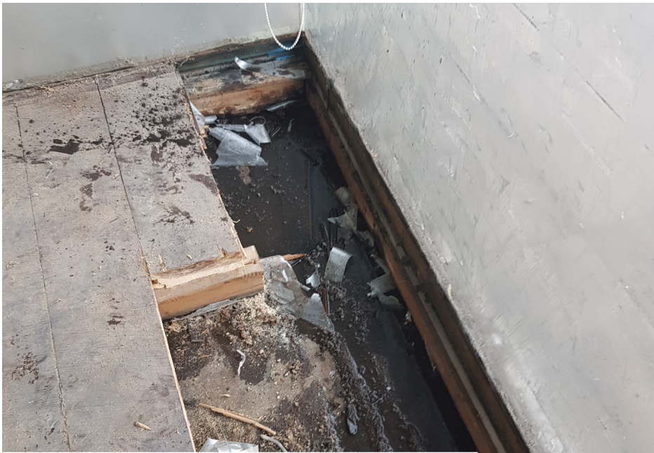
Carriage works interior - water ponding under floor boards
