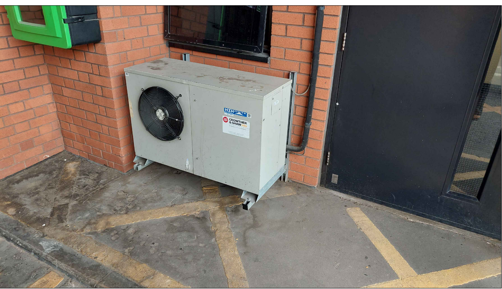
PHOTO 3 - EXISTING 1ND. COLD CONDENSER TO BE REPLACED FOR NEW. NEW SUPPORT FRAME SHALL BE INSTALLED IN THE SAME POSITIONS AS EXISTING.
