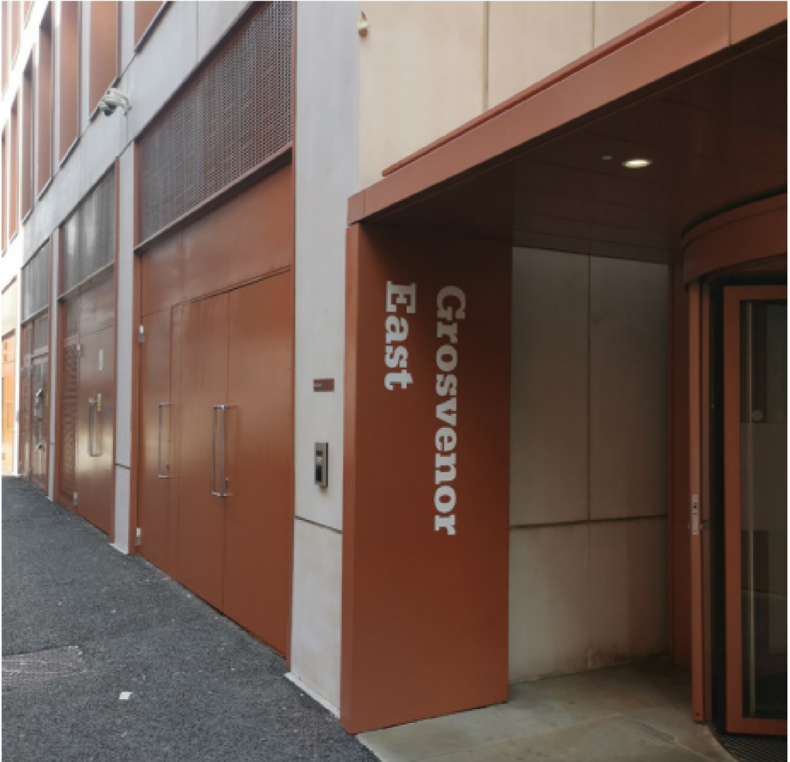
Replaced no sign
