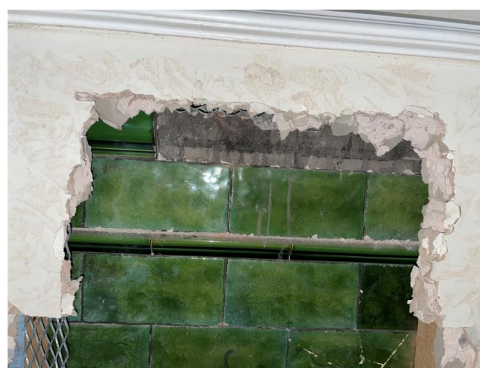
Fig. 14: typical details at 4 th floor showing missing tiling
