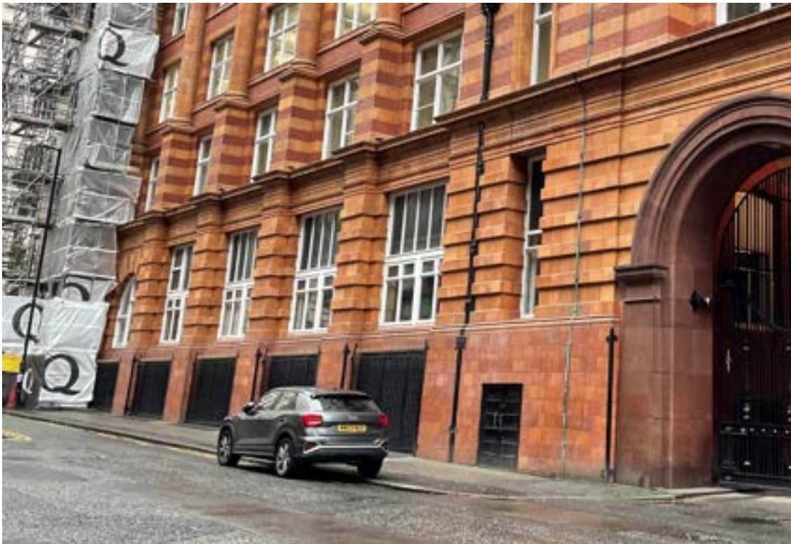
Figure 37: The Northern, Great Bridgewater Street elevation, showing the inserted c1950s and c1980s windows to the ground floor level.
