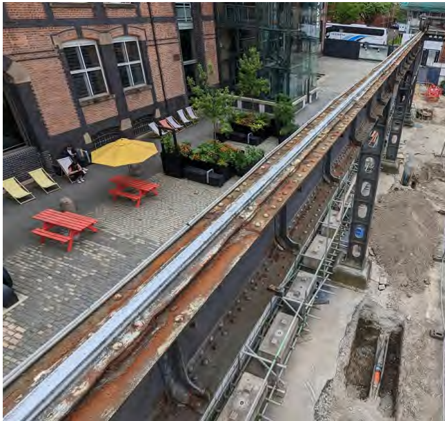
Figure 2-39 Typical corrosion to top face Gantry beam
