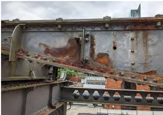
Figure 2-25 Corrosion to side face crane beam (eastern)
