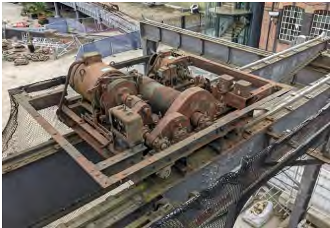
Figure 2-30 Lifting gear to western crane beam
