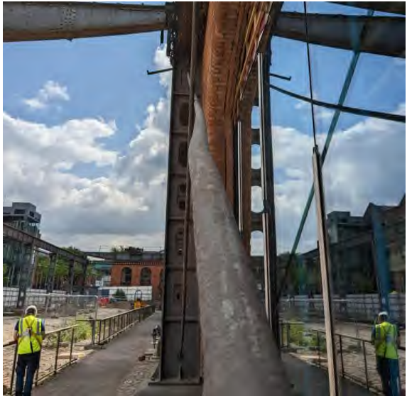
Figure 2-18 South cross bracing showing pitting & deformation
