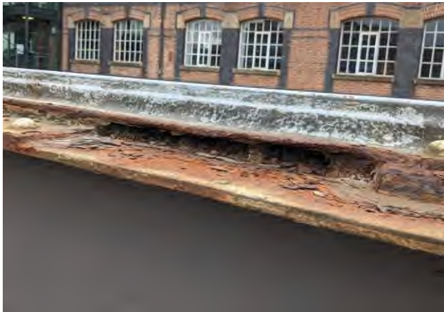
Figure 2-40 Moderate corrosion to top face Gantry beam
