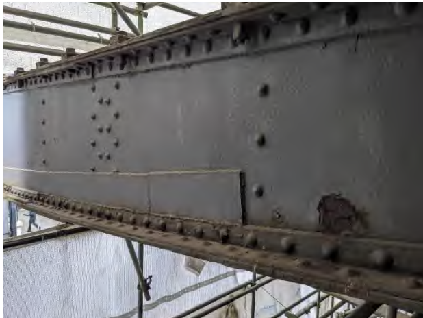
Figure 2-28 – Previous repair to crane beam
