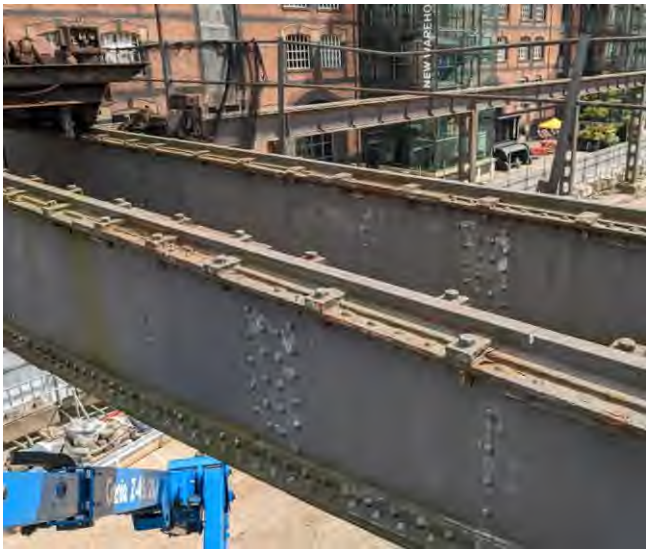
Figure 2-22 Corrosion to top face crane beam
