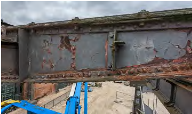
Figure 2-24 Corrosion to side face crane beam (western)
