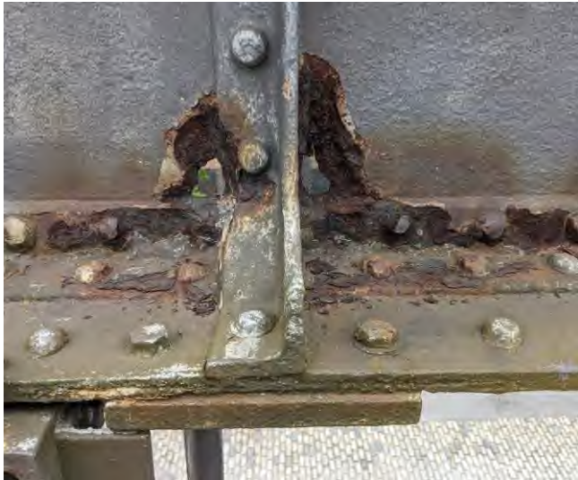
Figure 2-37 Severe corrosion to Gantry beam at stiffener
