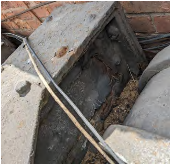
Figure 2-27 Crane beam end corrosion
