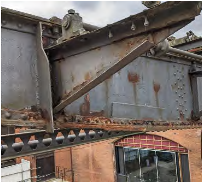
Figure 2-26 Corrosion to bottom of crane beam
