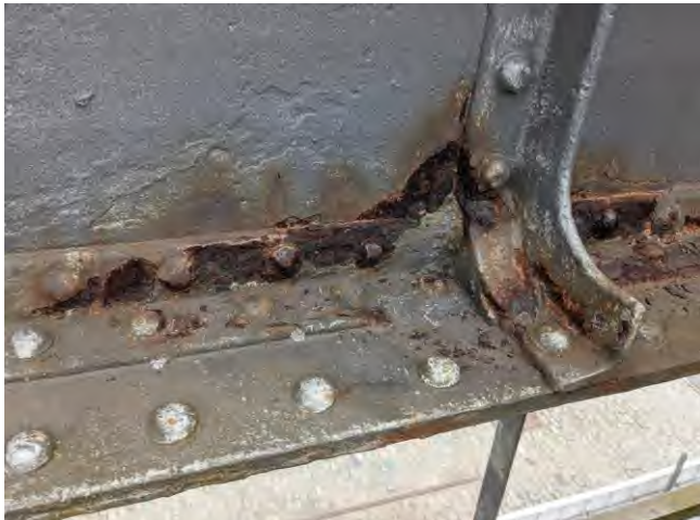
Figure 2-36 Typical corrosion to Gantry beam at stiffener
