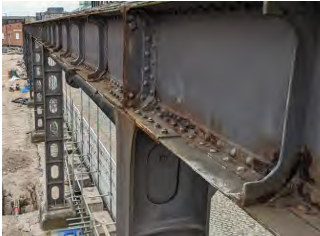
Figure 2-38 Typical corrosion to Gantry beam
