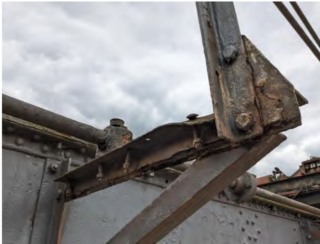
Figure 2-29 Crane beam balustrade – corrosion & deformation
