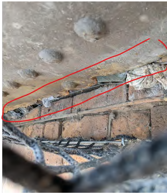
Figure 2-31 Severe corrosion & loss of section width – southern face of south Gantry beam, bottom flange
