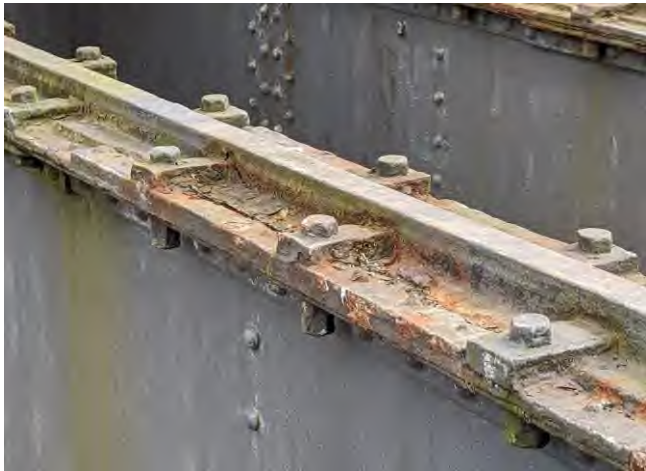
Figure 2-23 Corrosion top face crane beam
