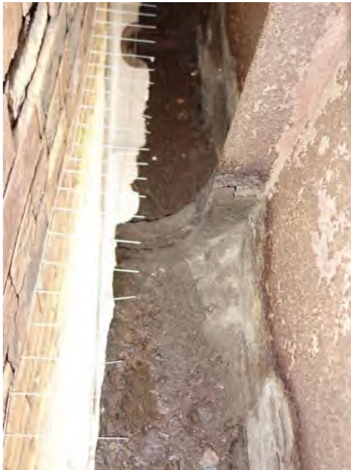
Figure 2-34 Corrosion and lack of protection to southern face of south Gantry beam
