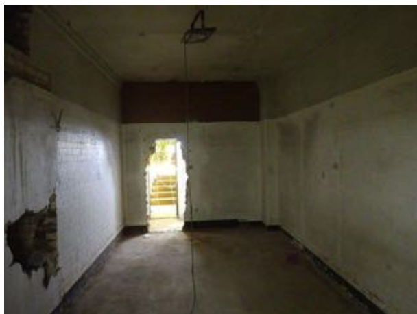
Photo B7 of Walk in Fridge
