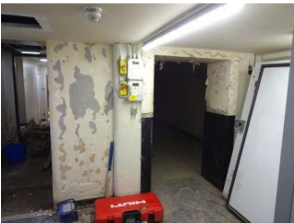
Photo B9 of Walk in Fridge
