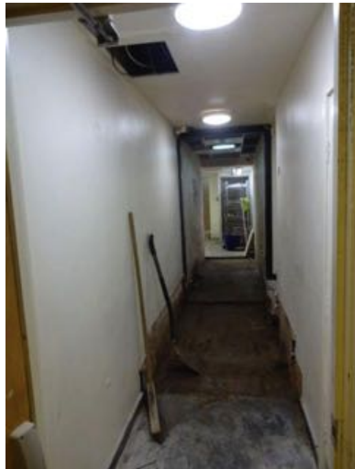
Photo B10 of Corridor Wall
