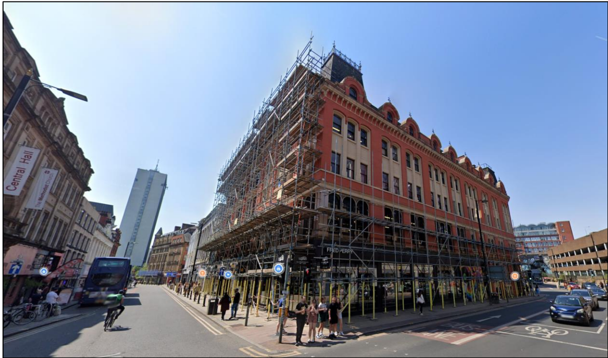
Fig 3: Example of negative visual impact of scaffolding on the street scene at 41-43 Oldham Street
