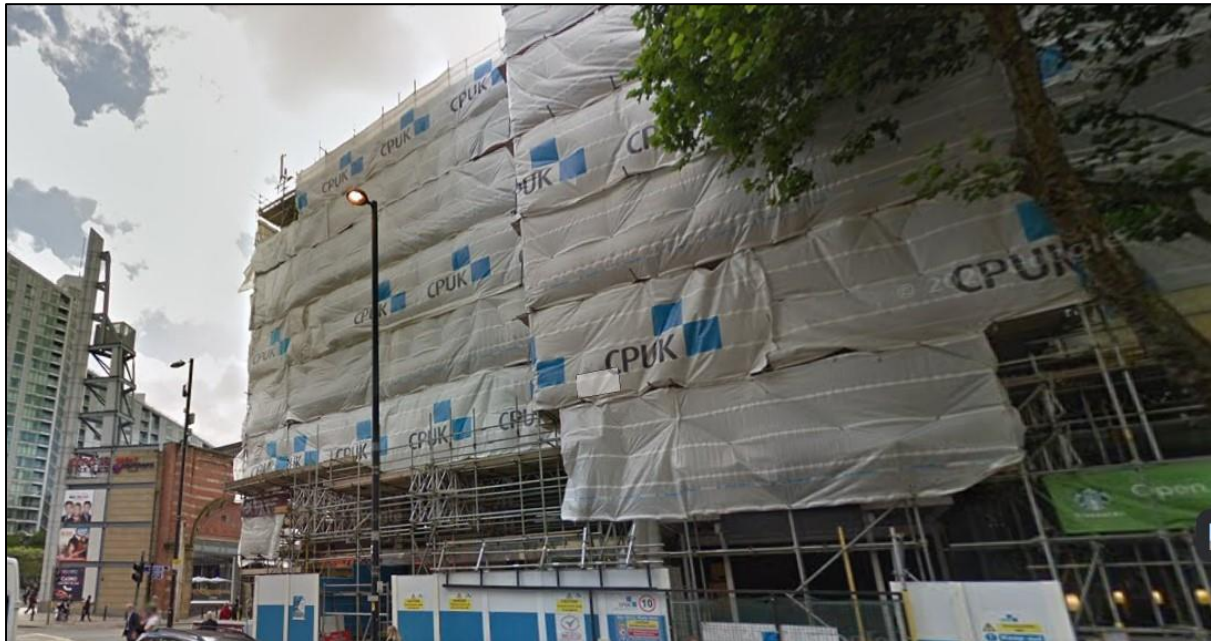
Fig 4: Example of negative visual impact of scaffolding on the street scene at 11 Quay Street
