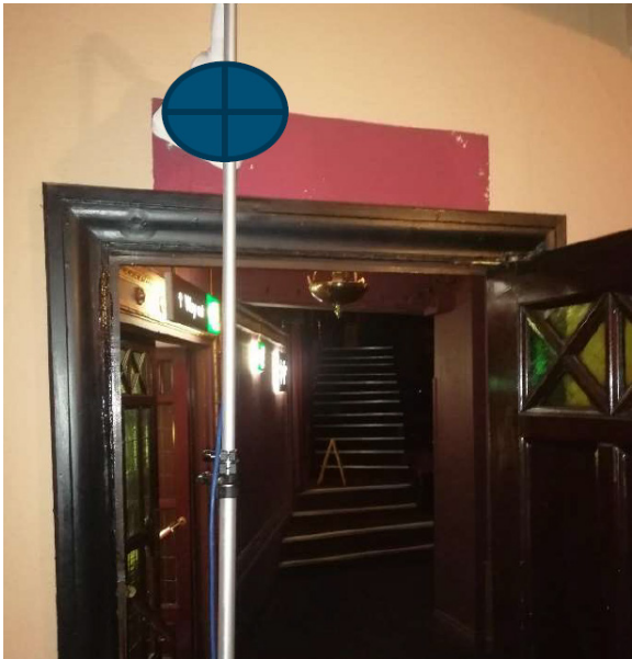
Location AP 32 - Circle Floor one - Unit is at high level and centered on the door in low prominence location.
