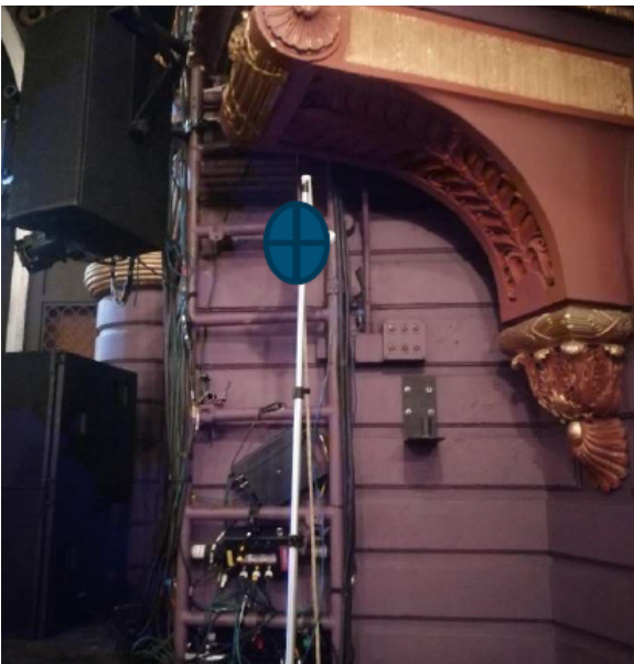
Location AP A3 - Stalls level - unit installed discreetly within existing cluster of electrical units.
