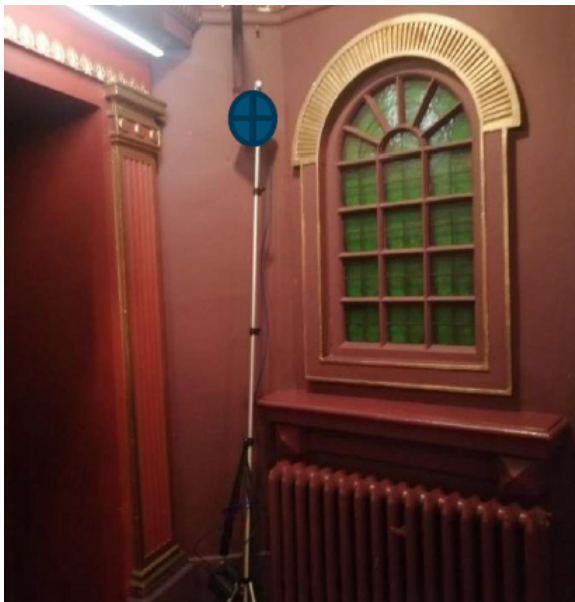
Location AP A13 - Stalls level - unit installed symmetrically on blank wall between architraves
