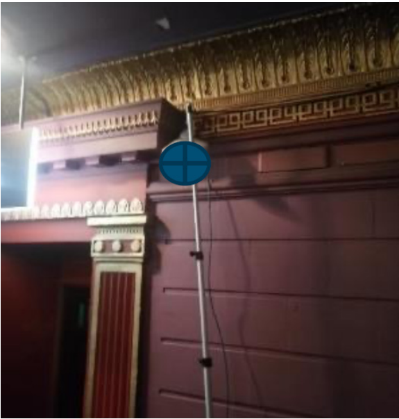
Location AP A5 - Stalls level - unit fixed discreetly adjacent to cornicing and in close proximity to existing conduit.
