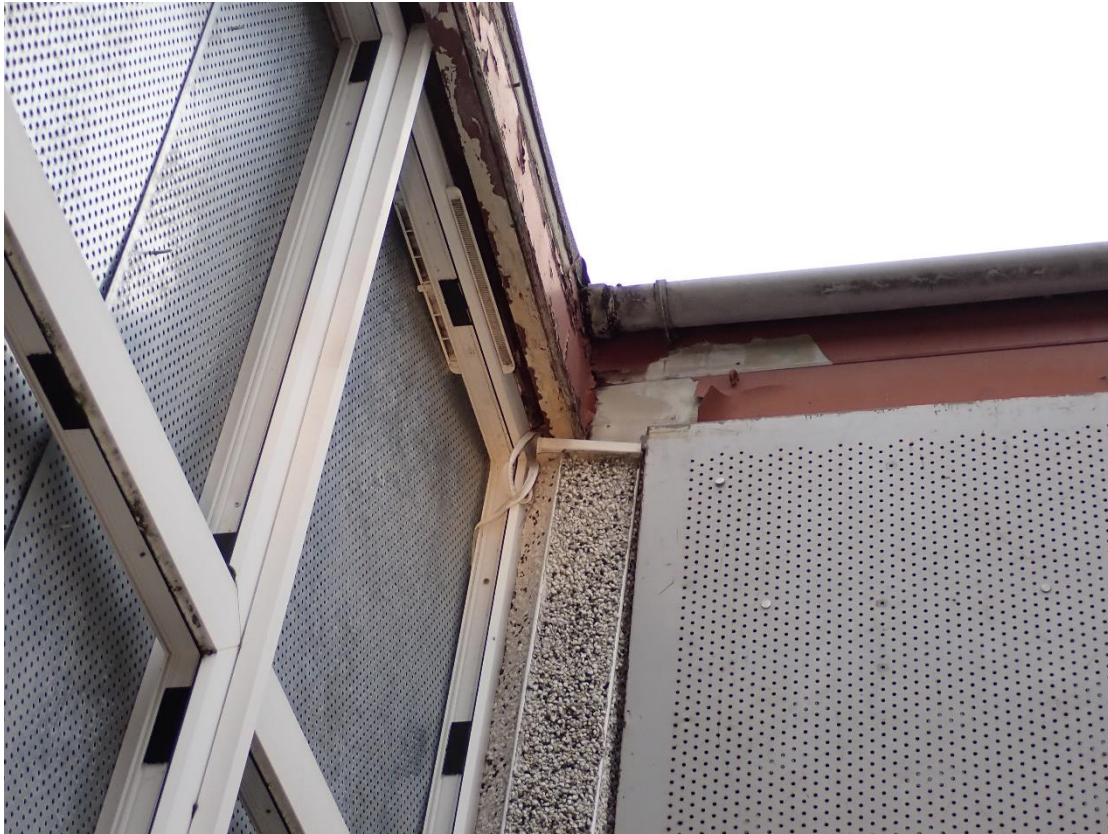
Photograph 5. Gap under the bargeboard on the southern aspect of the central corridor.
