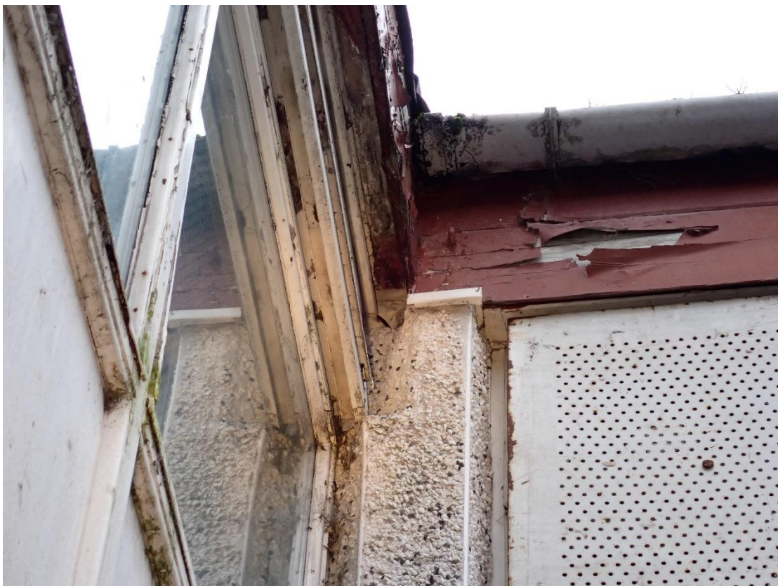
Photograph 6. Gap in the bargeboard on the northern aspect of the central corridor.
