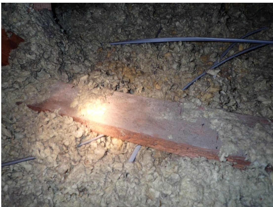
Photograph 12. Mouse droppings identified in the loft space of Flat 9.
