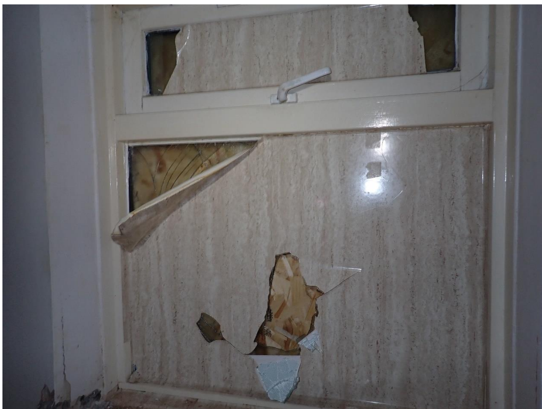
Photograph 15. Wooden boards behind a window in Flat 1.
