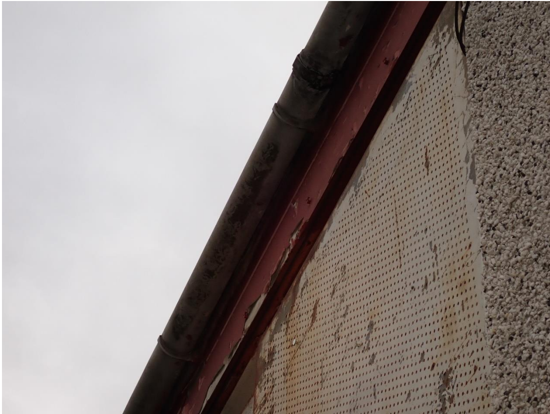
Photograph 3. Potential roosting feature where the wooden bargeboard meets the underside of the roof tiles, behind the drainpipe.
