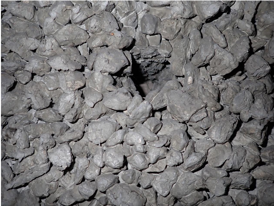
Photograph 13. A hole in the south internal stone render wall in the loft space of Flat 11.
