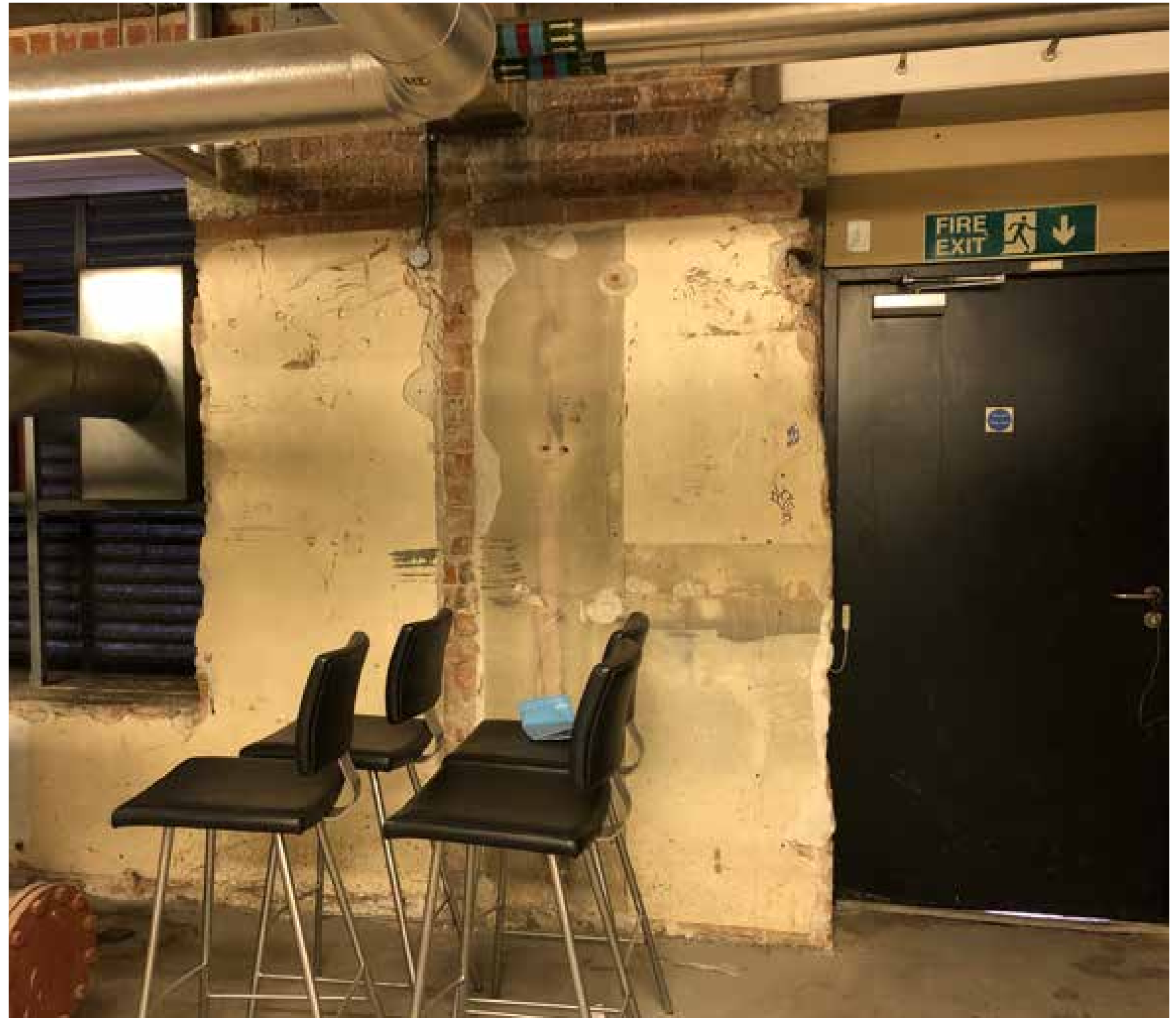
Photograph of existing boiler room, including existing louvre to the left of image, and existing door to the right of shot.
