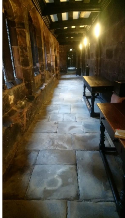
College House Baronial Hall Corridor – Stone floor condition.
