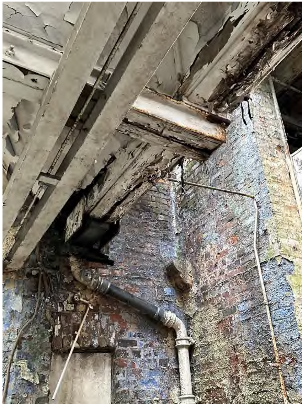
Figure 69 – Continued water ingress leading to timber decay and failure (taken 2023)
