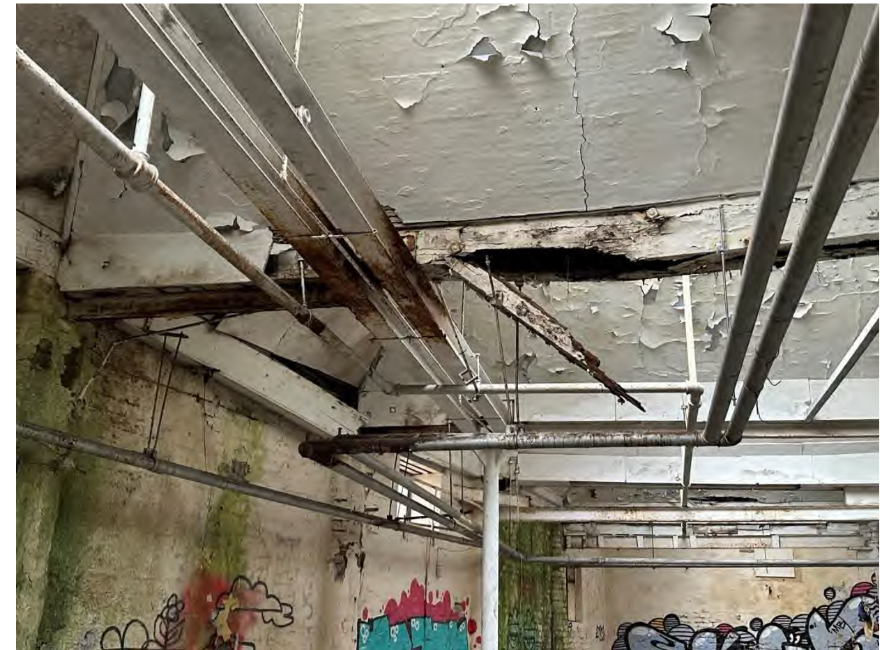
Figure 68 – Evidence of continued water ingress and staining (taken 2023)
