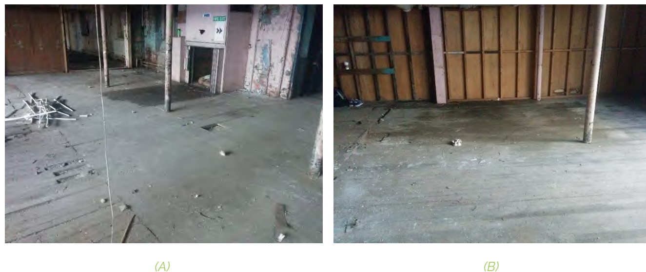
Figure 58 - Water ingress at ground floor and missing timber floorboards (taken 2018)
