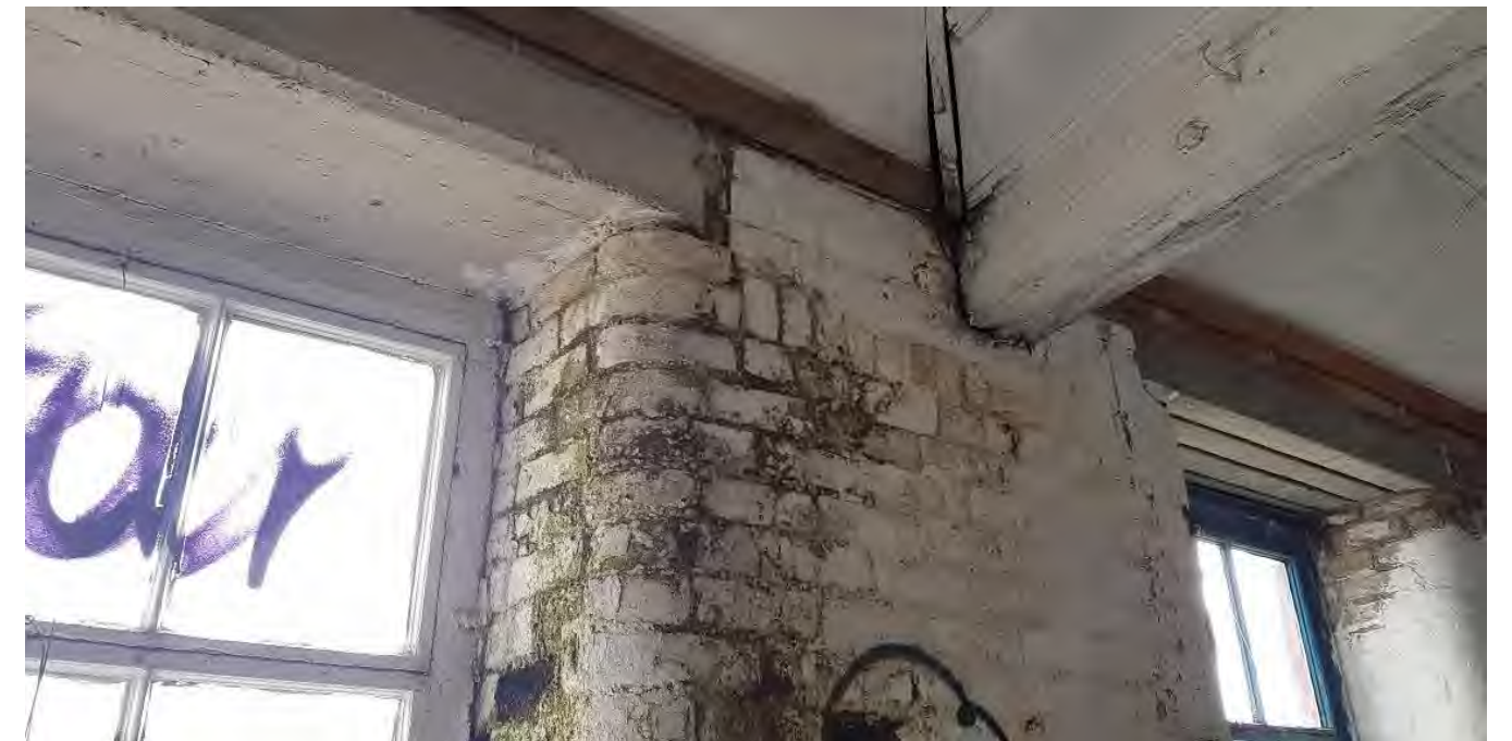
Figure 22 - Internal vegetation growth on southern masonry wall (taken 2018)
