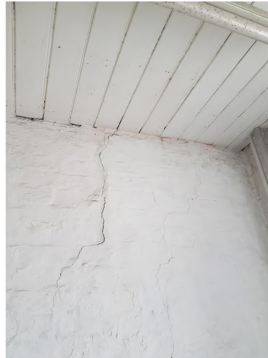
Figure 31 - Cracking to wall elevation on Cambridge Street (taken 2018)
