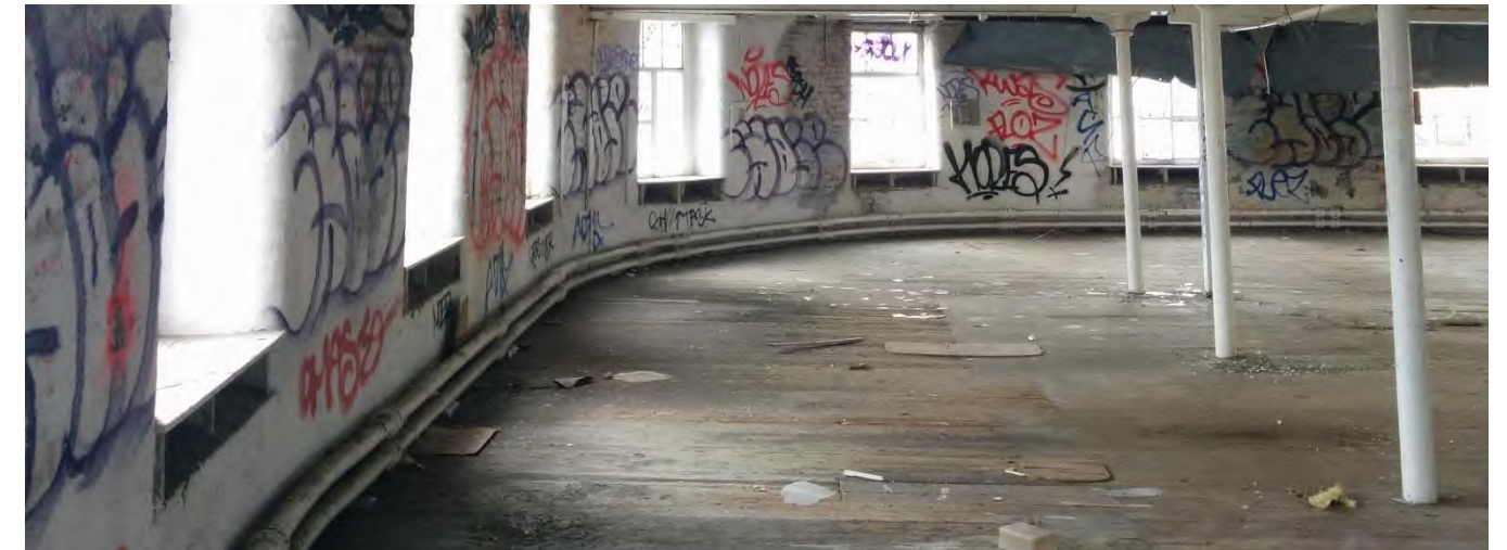
Figure 21 - Deterioration of the timber floor at third floor level (taken 2018)
