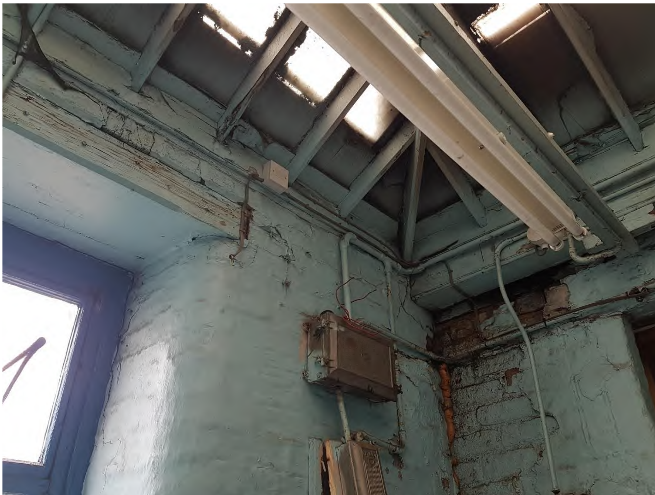
Figure 23: Debonding of walls between 1882 warehouse and 1801 mill (taken 2018)
