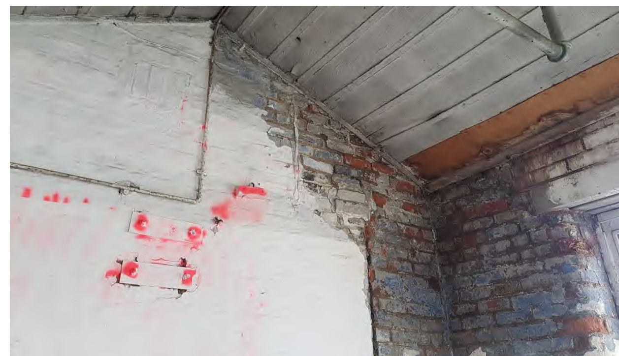
Figure 19 - Cracking to external wall on Cambridge Street, corresponding to return wall (taken 2018)
