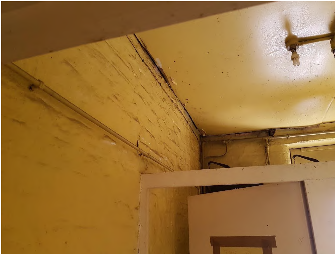
Figure 28 - Further cracking through external wall (taken 2018)
