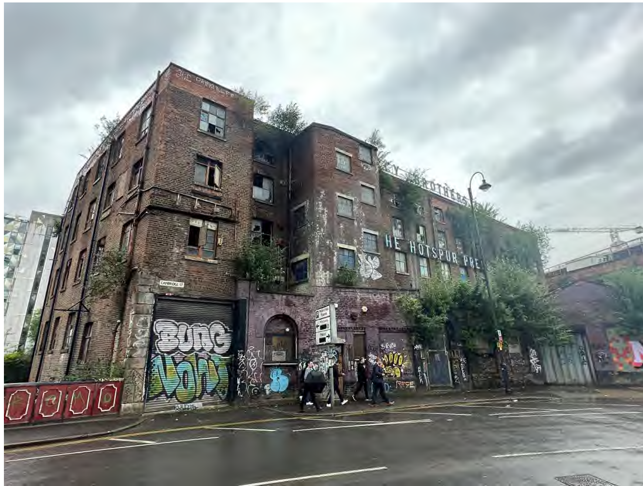
Figure 86 - Severe vegetation growth on eastern elevation has continued since previous survey (taken 2023)
