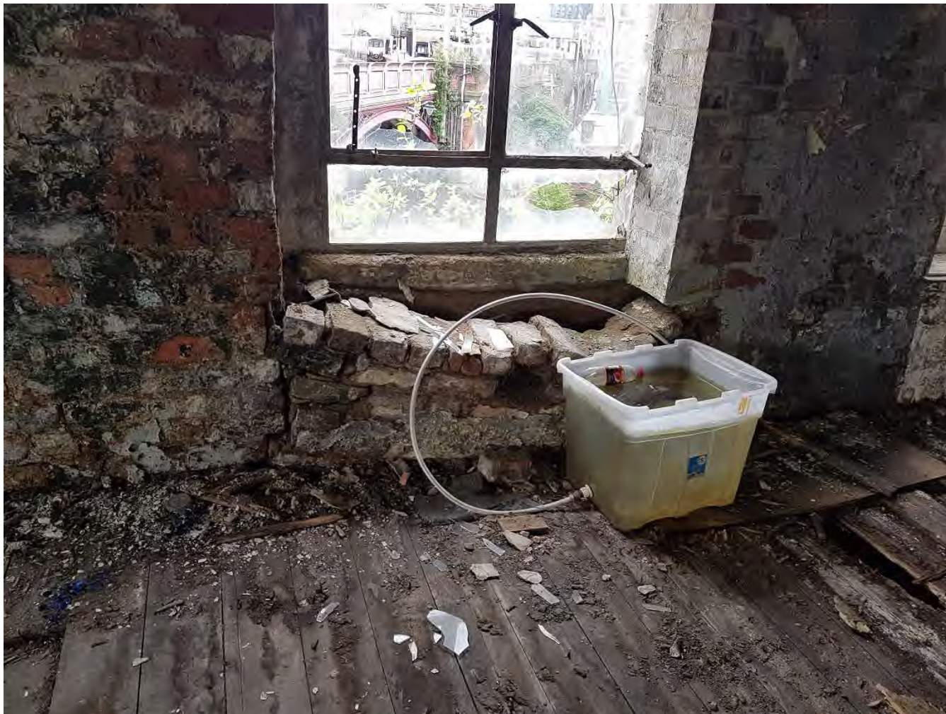
Figure 45 - Significant movement of sill at third floor level. Also shows water ingress (taken 2018)
