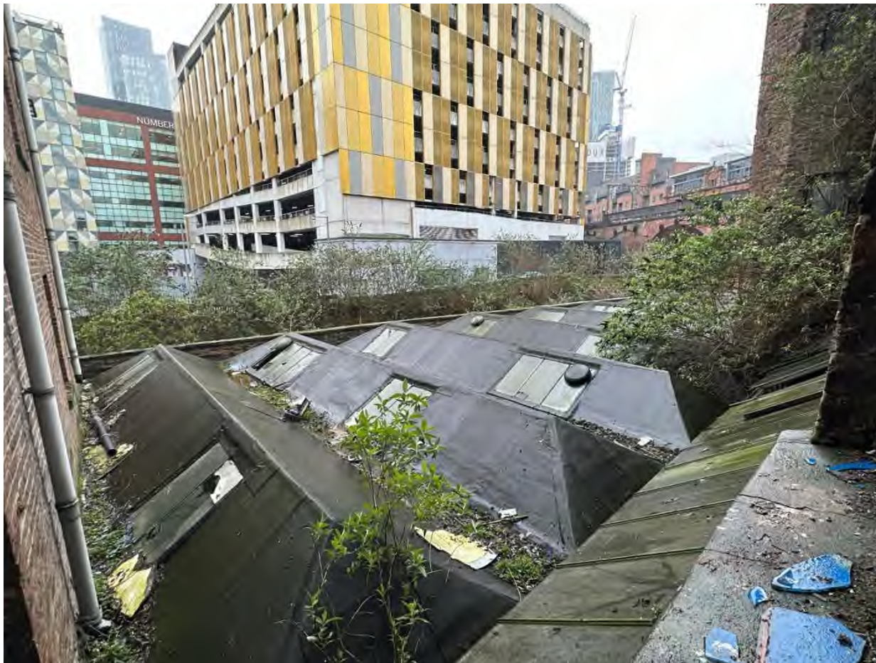
Figure 67 – Roof and continued vegetation growth in gutters (taken 2023)
