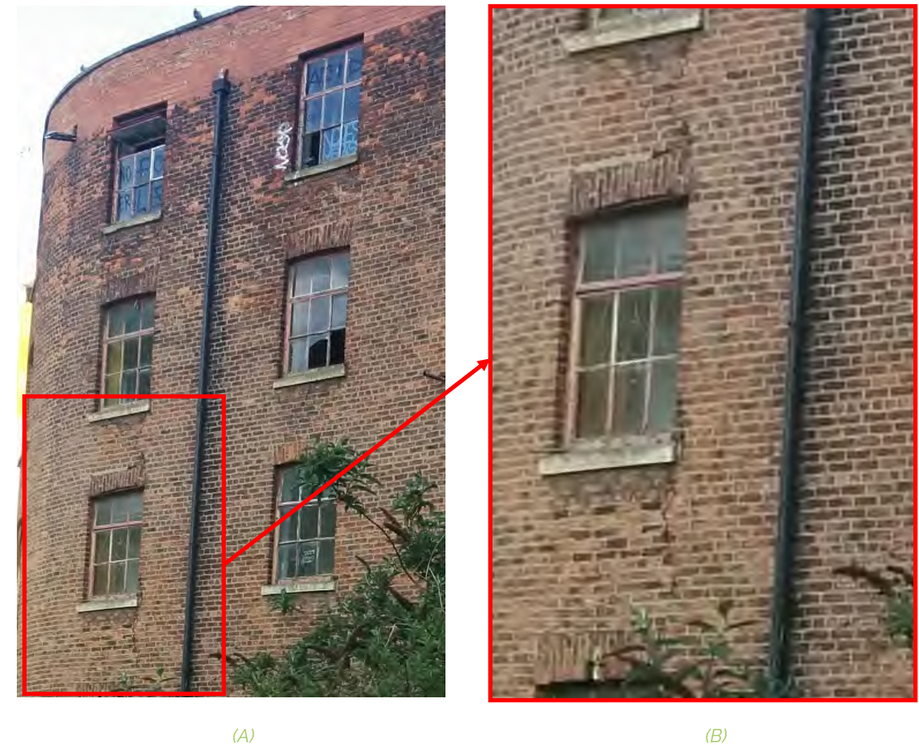
Figure 78 - Significant cracking on southern elevation (taken 2018)
