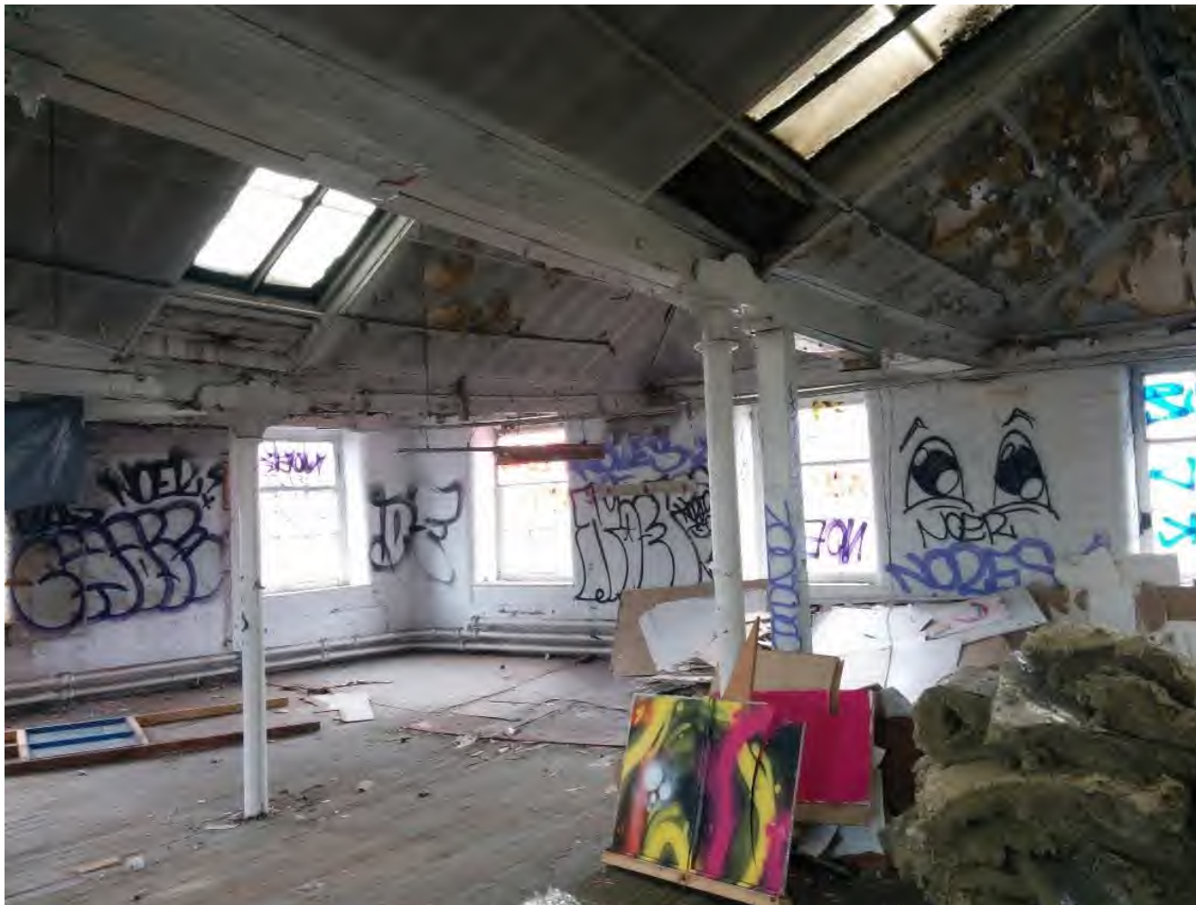
Figure 20 – Significant dish to the third floor (left column) (taken 2018)
