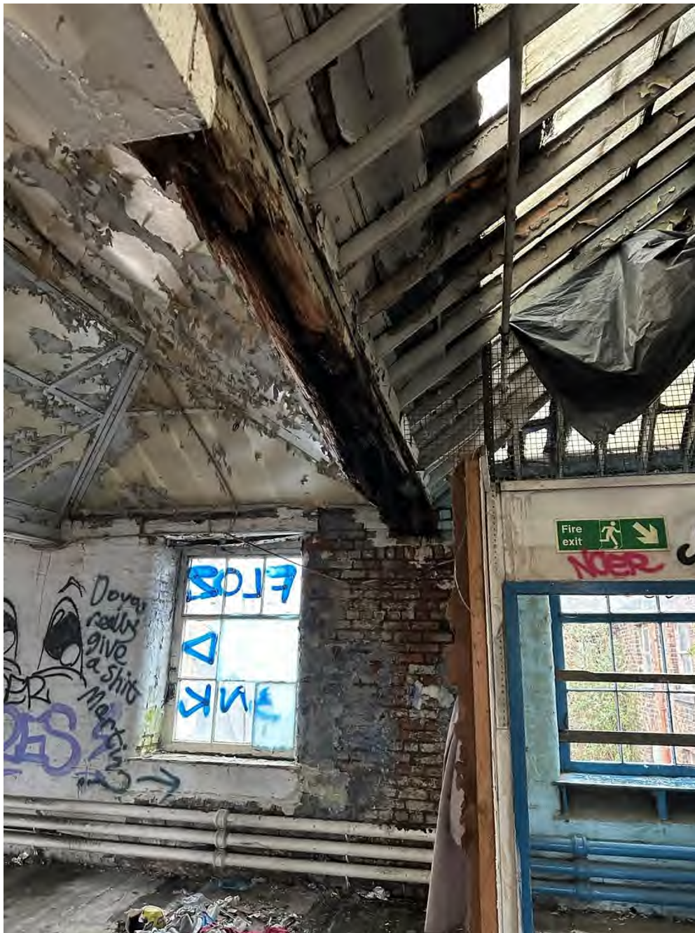
Figure 13 – Timber structural member decay and section loss (taken 2023)
