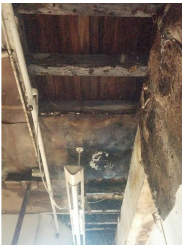
Figure 54 - Very damp timber floor areas (possible rot) at first floor level (taken 2018)
