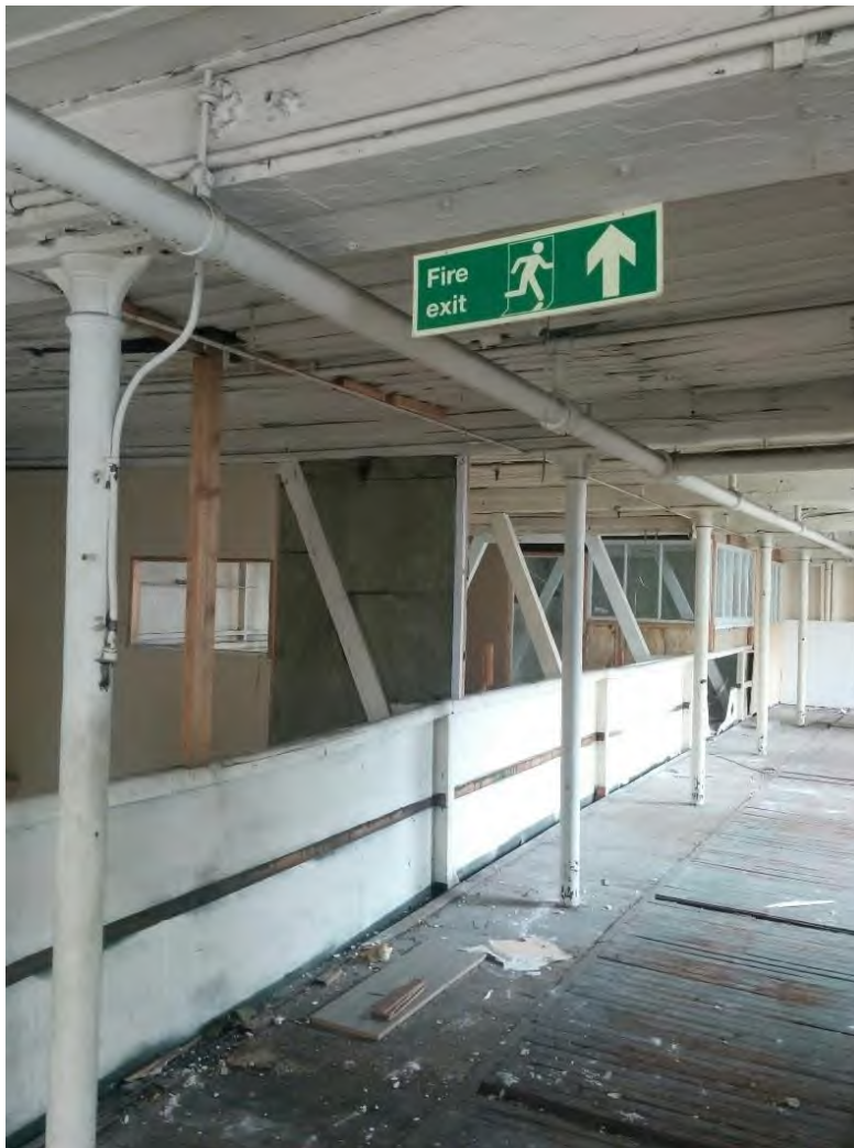
Figure 49 - Damp timber floor with missing floorboards at second floor level (taken 2018)
