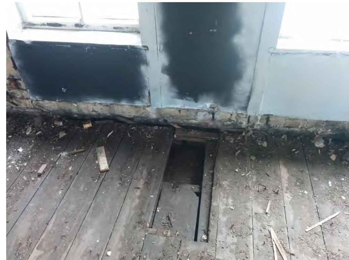
Figure 46 - Missing timber floorboards at third floor level (taken 2018)
