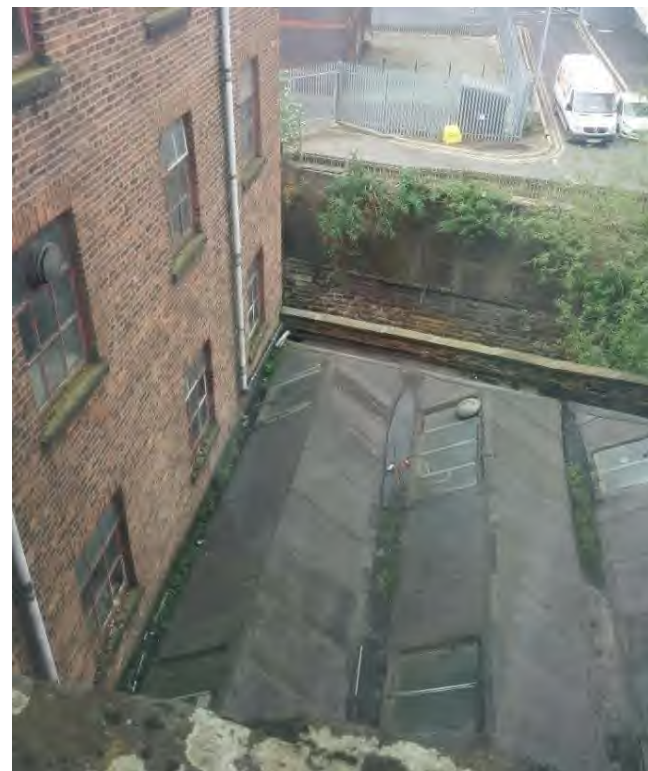
Figure 63 - Roof and vegetation growth in gutters (taken 2018)
