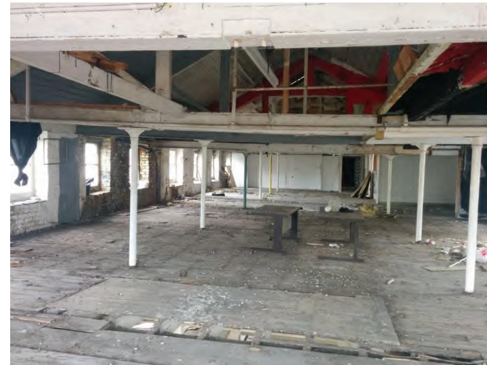
Figure 41 - Cast iron columns supporting timber roof trusses; damp timber floor at third floor level (taken 2018)
