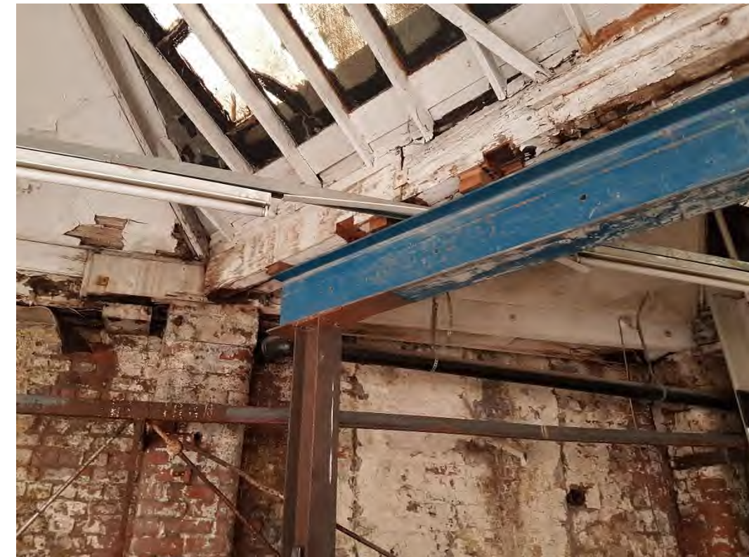
Figure 72 - Steelwork portal frames supporting decayed timber roof beams (taken 2018)
