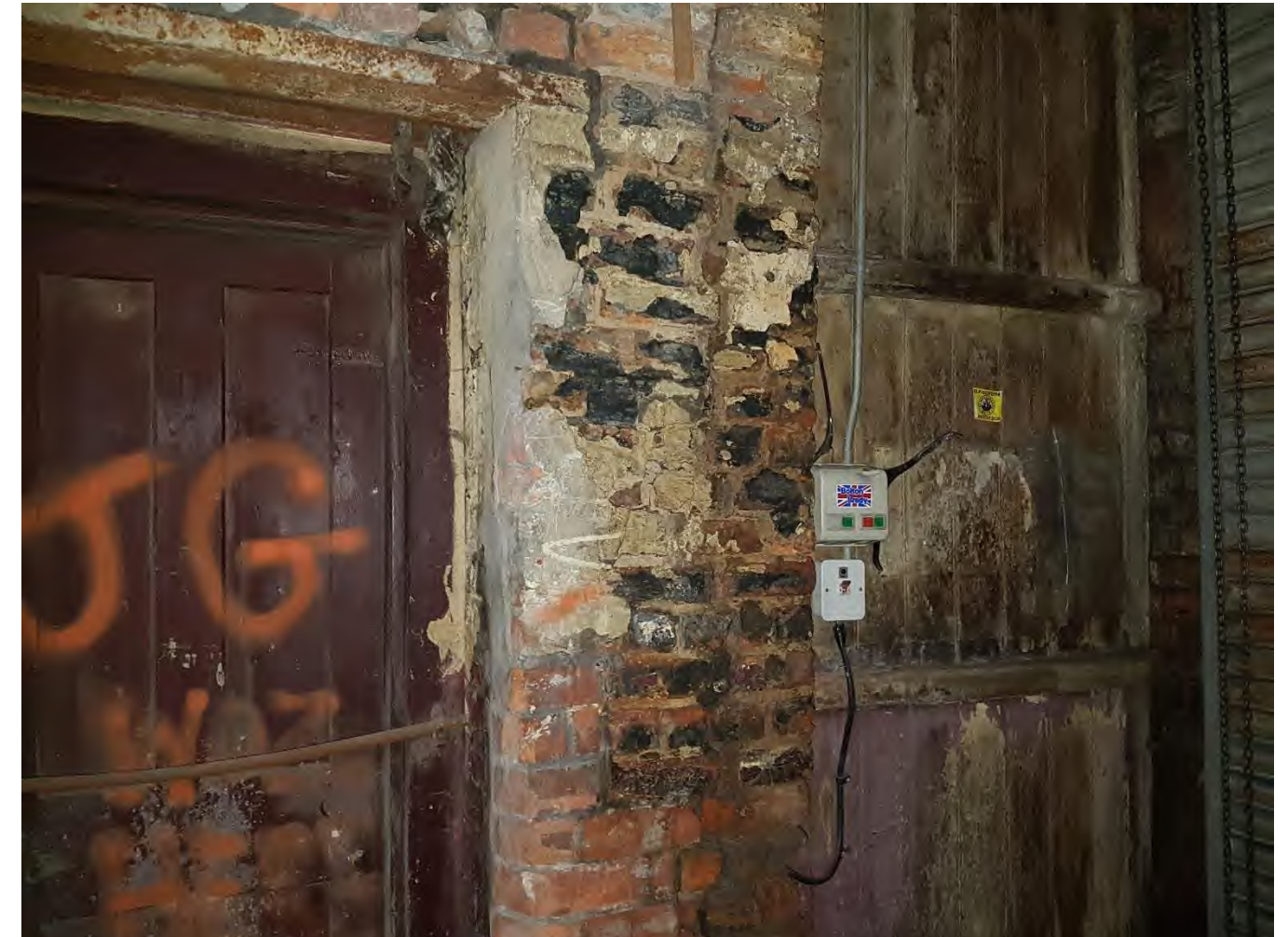
Figure 36 - Extensive cracking through pier at ground floor level (taken 2018)
