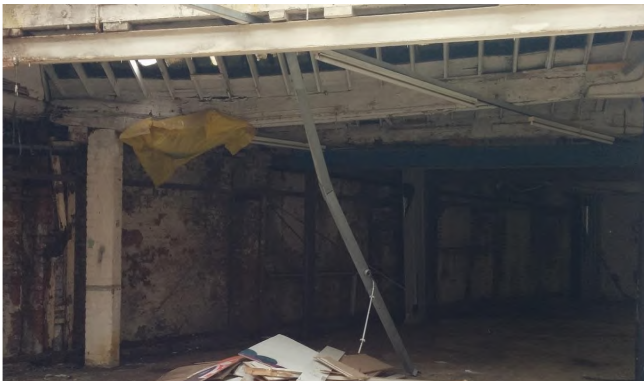
Figure 74 - Failed timber beam end (taken 2018)
