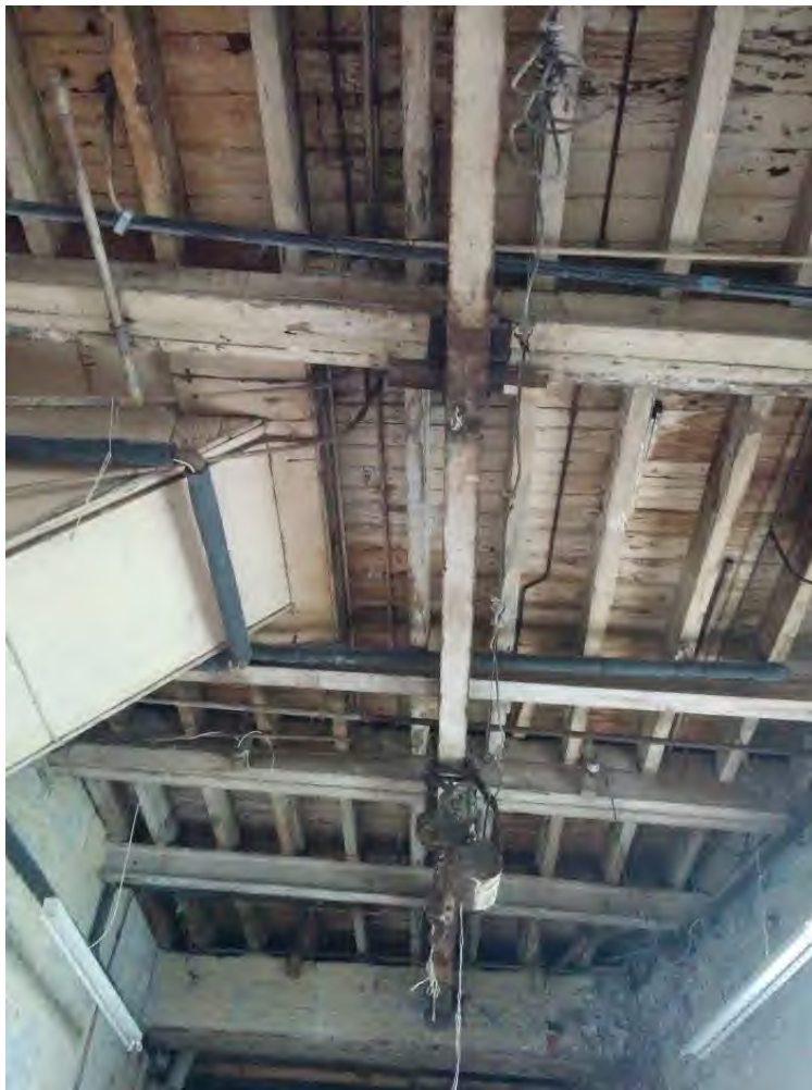
Figure 30 - Corroded steel beams infilled with brickwork (far end) (taken 2018)
