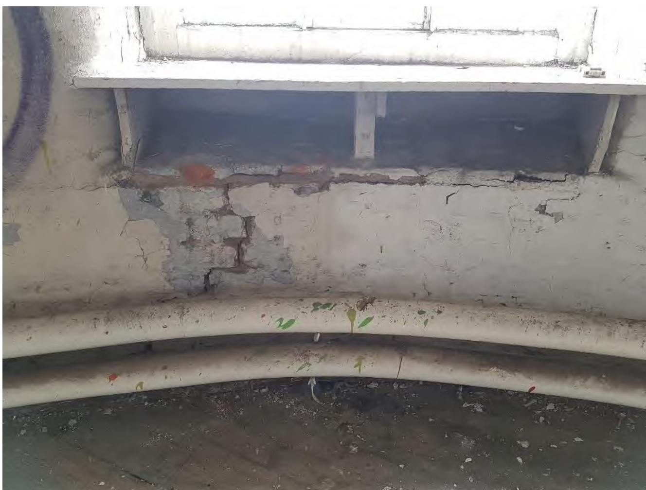
Figure 17 - Cracks below sill at third floor level (taken 2018)
