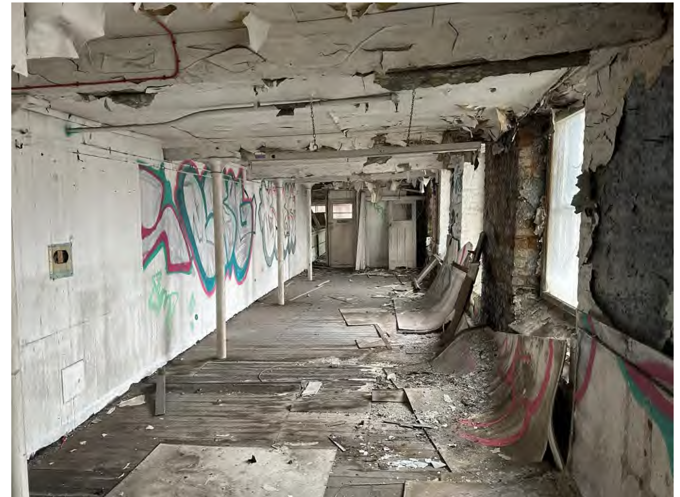
Figure 50 – General view of second floor showing deterioration due to continued water ingress (taken 2023)
