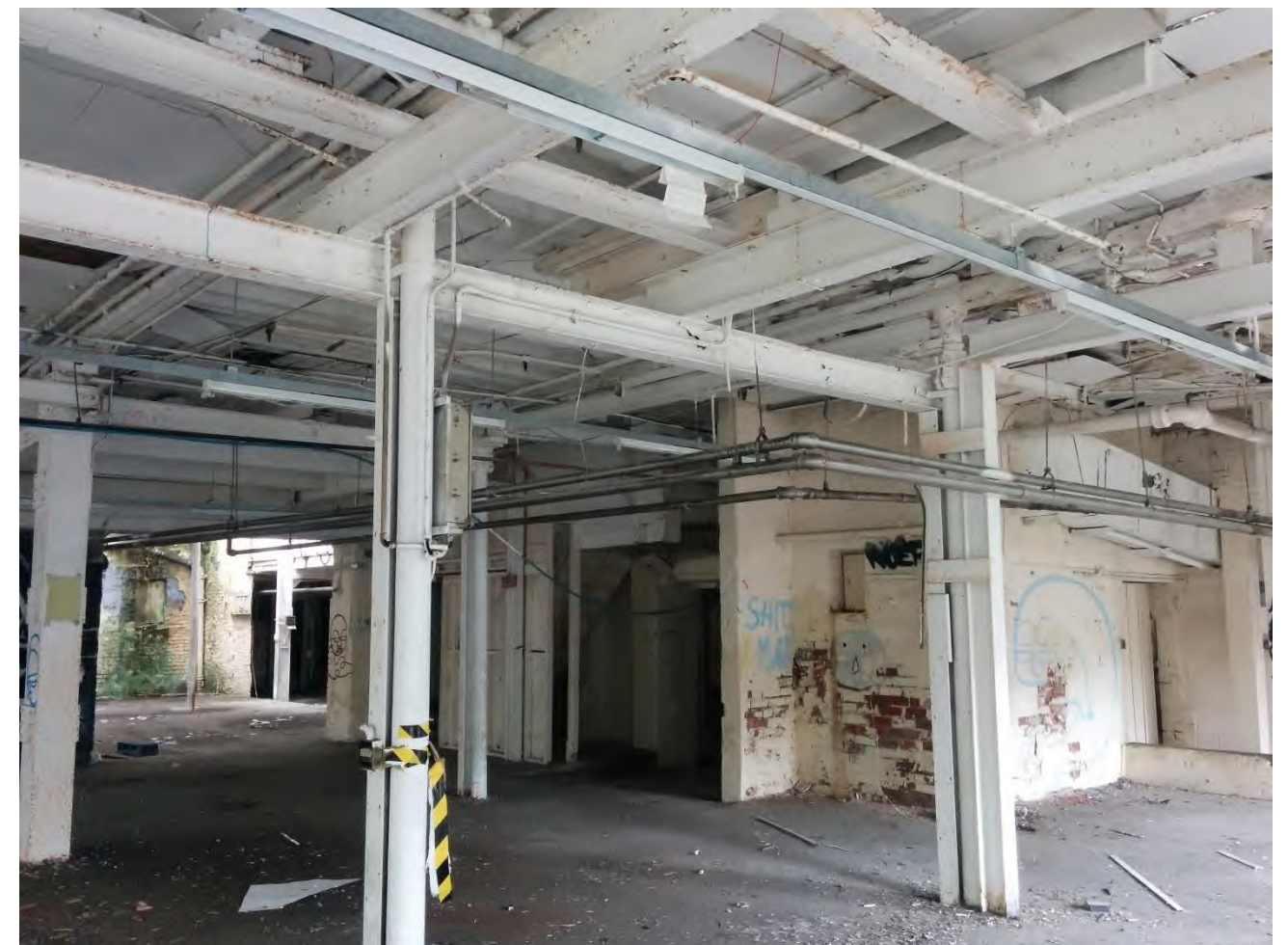
Figure 38 – Ad hoc additional steel columns in basement (taken 2018)
