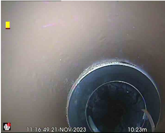
9_SVPB_FW10B.jpg, 00:01:04, 10.23 m Broken pipe at joint from 4 o'clock to 5 o'clock, SMALL PEACE OF PLASTIC STICKING OUT AT JOINT
