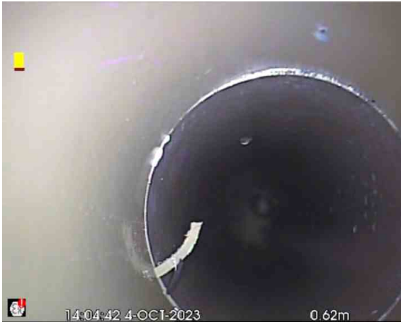
89_SW 3A_MAIN.jpg, 00:00:09, 0.62 m General remark, PLASTIC WEDGED IN JOINT
