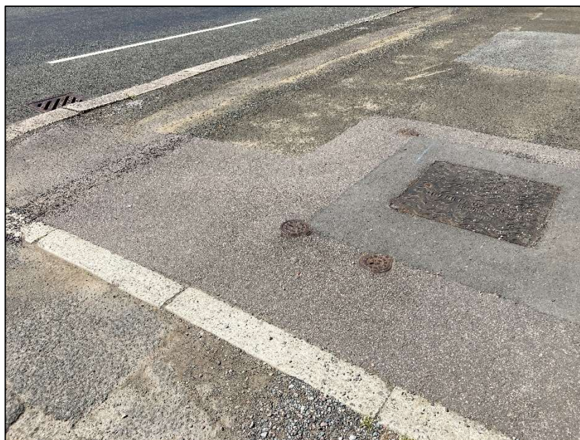
Figure 17 Inspection chambers located near to road.
