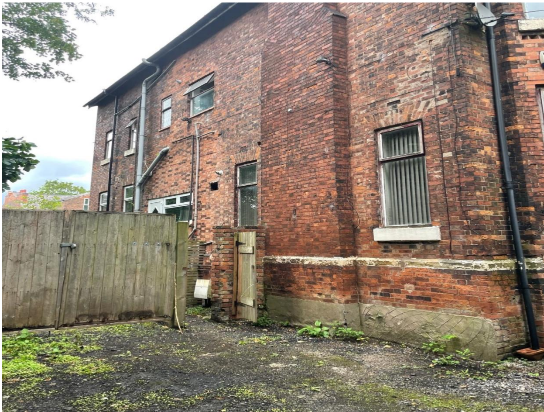
Image 3 – Photograph of side elevation from driveway – note the general untidy nature of site and brickwork/detailing in need of restoration.
