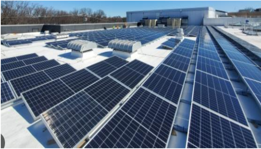
Figure 34 - Roof Mounted Photovoltaic Panels
