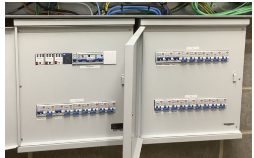
Example of an installed Array Controller and additional Distribution Board
