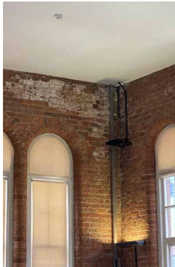
Water ingress to first floor
