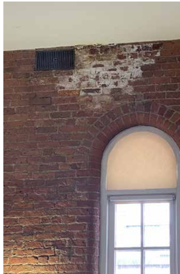
Water ingress to first floor
